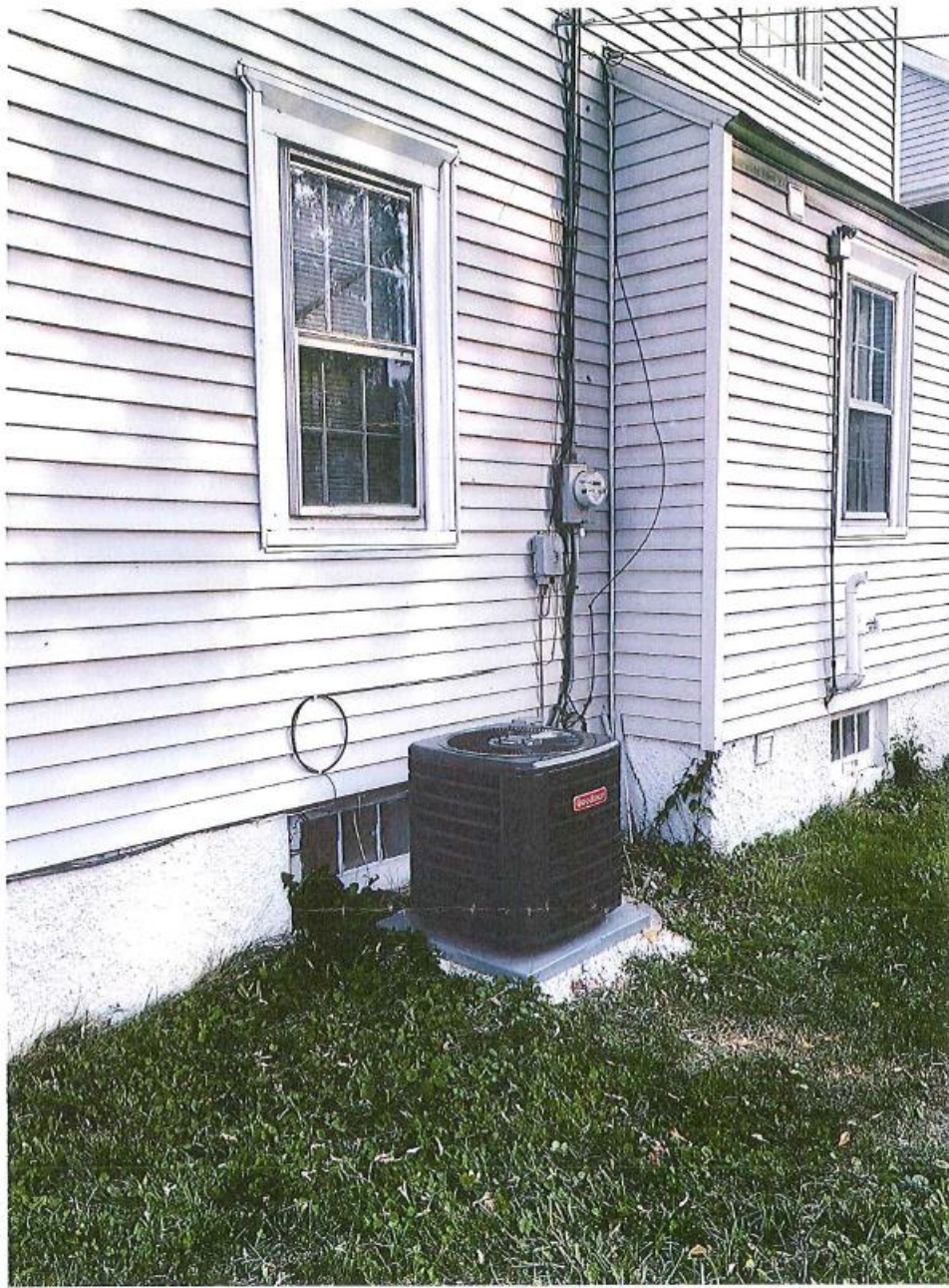
Photo of a/c unit location
