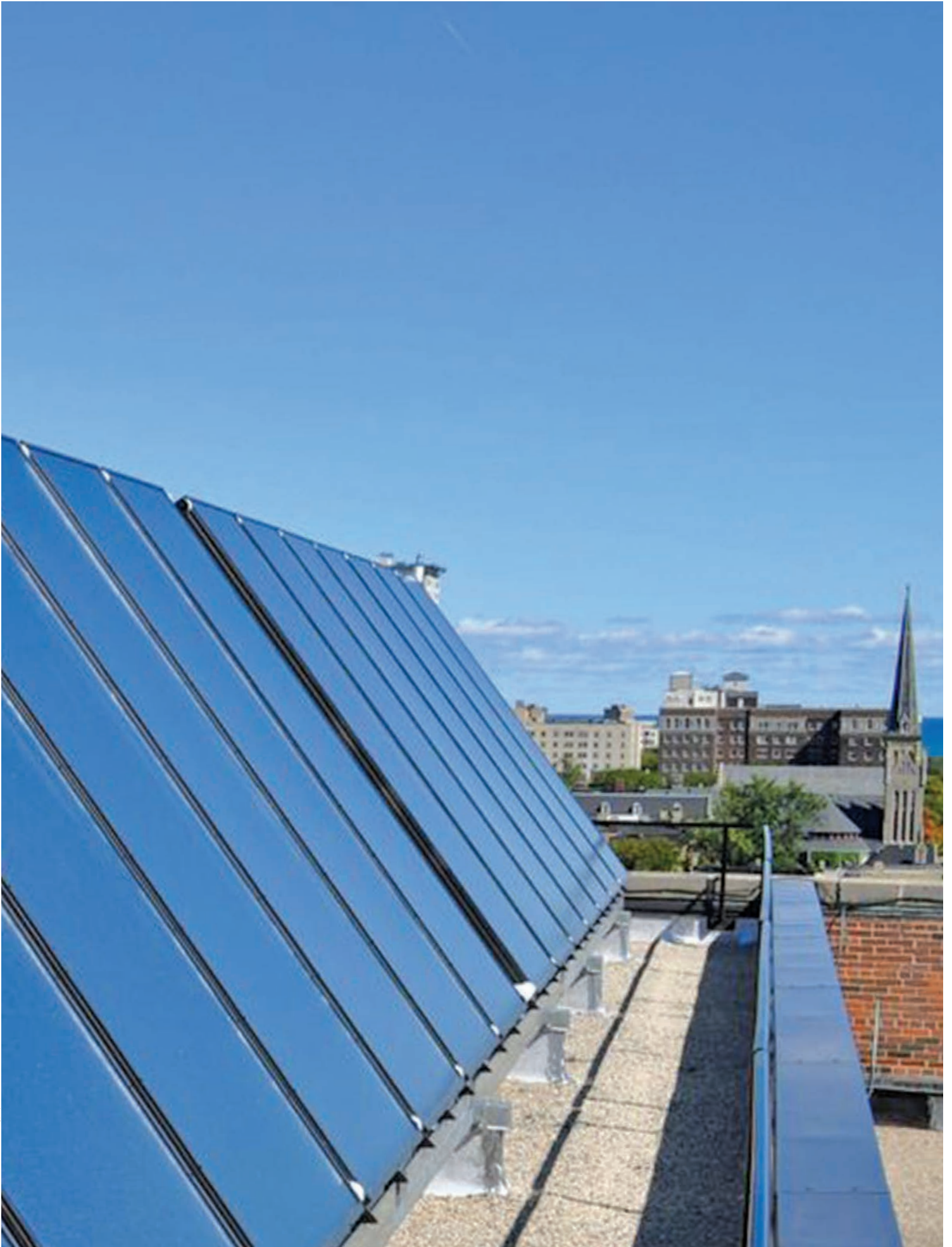
Solar at MSOE. Photo: H&H Solar Energy Systems
