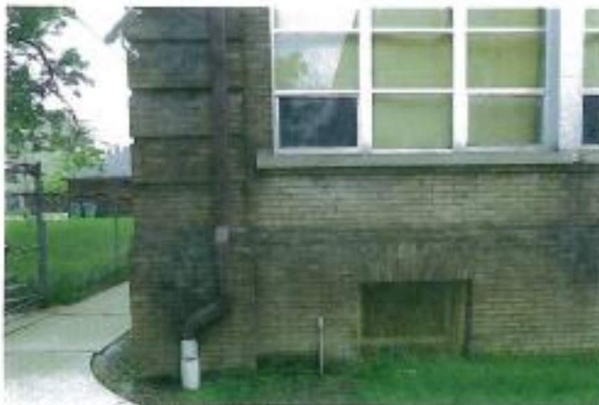
FIGURE 26: Severe deterioration of brick and mortar at northeast corner from rising damp caused by the moisture saturated and flooded basement/foundation conditions. Algal growth is also typical in this area.
