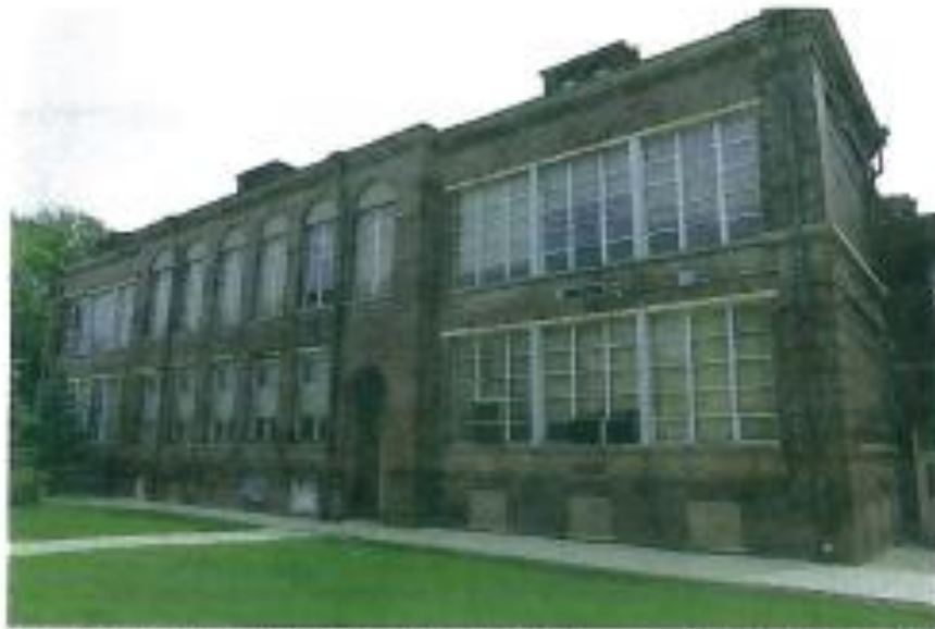
FIGURE 25: View looking southeast. Connection to Rincker Library appears at right. Discoloration at the building base due to rising damp from excess water infiltration.
