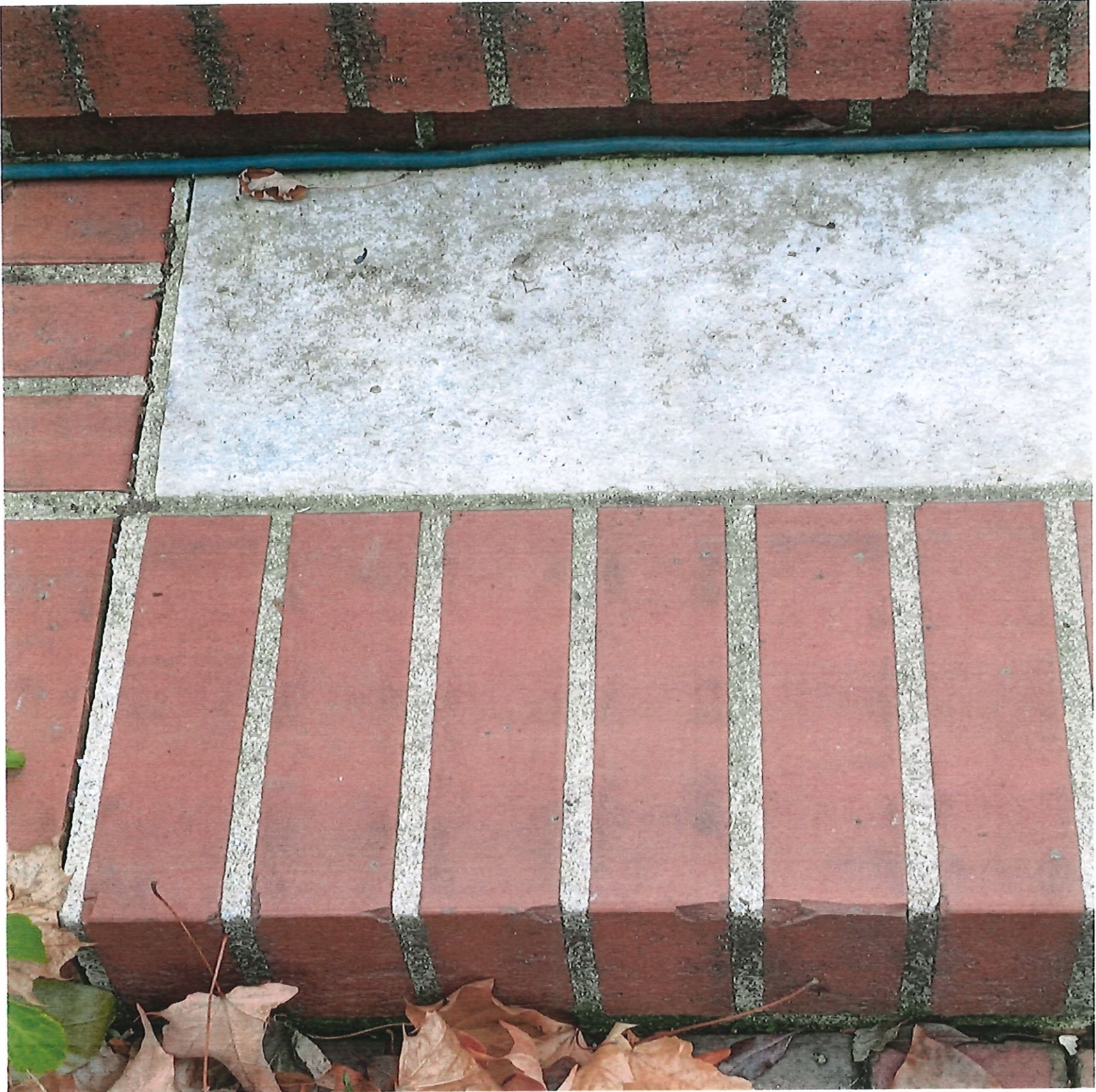
Front stoop settled; mortar needs repair/maintenance
