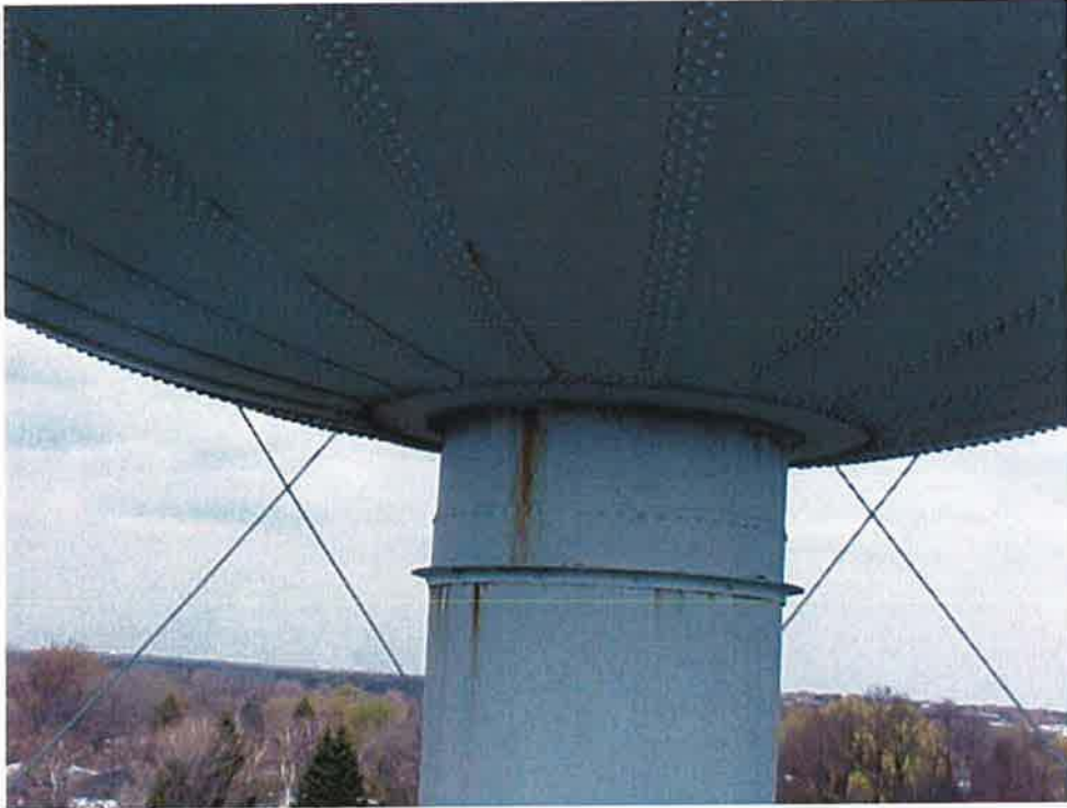
Fig. 3 Elevated Storage Tank Leak Location
