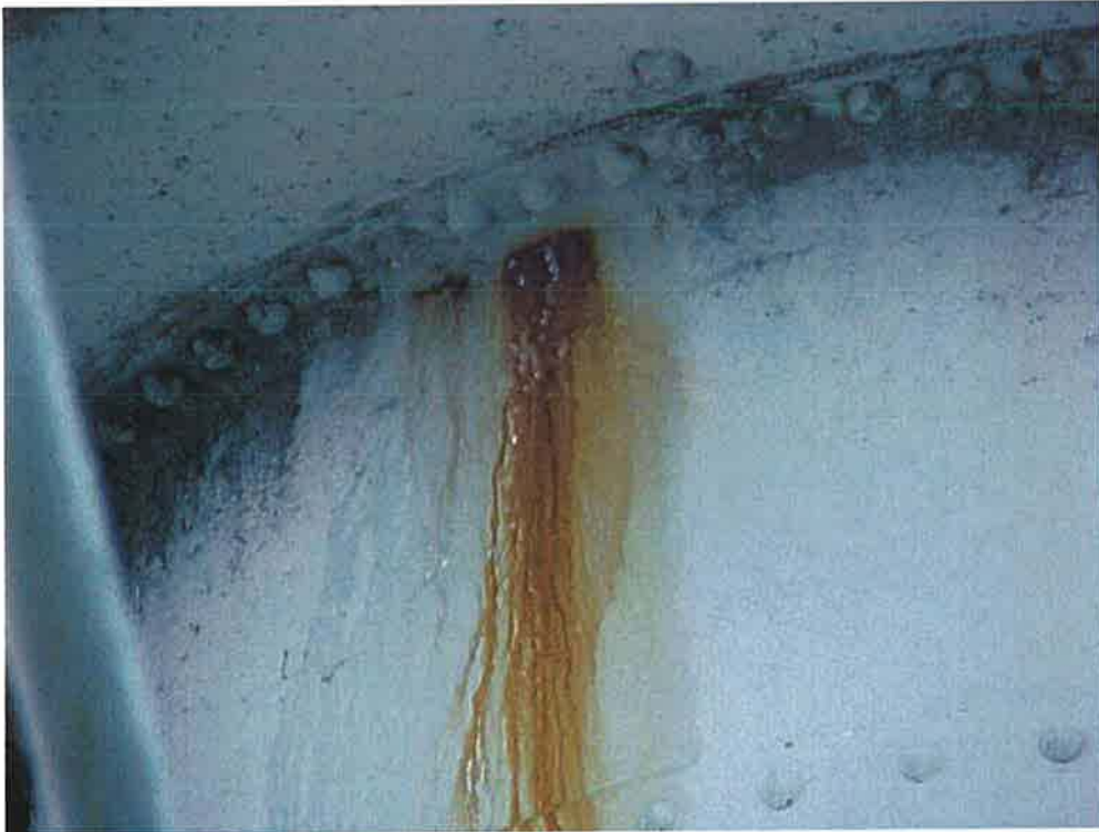
Fig. 4 Elevated Storage Tank Leak
