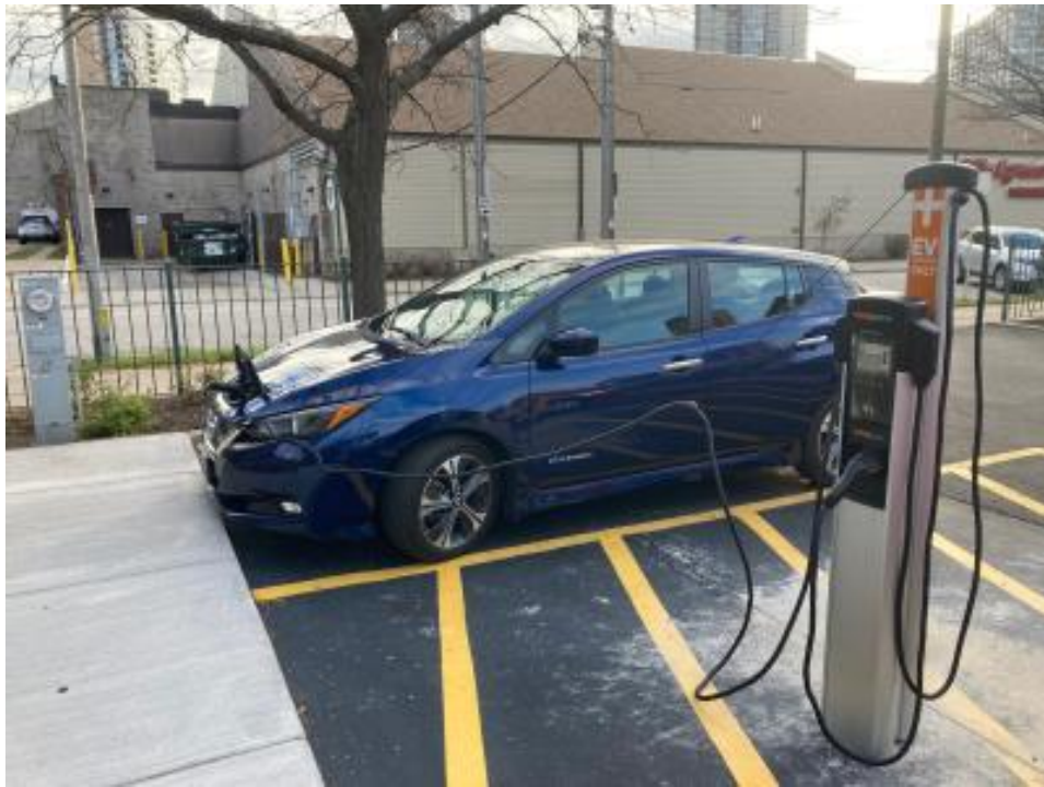
Electric vehicle charging
