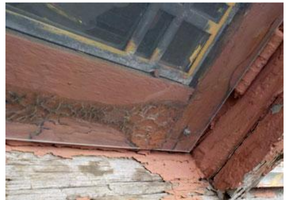
Lead paint chipping from a window
