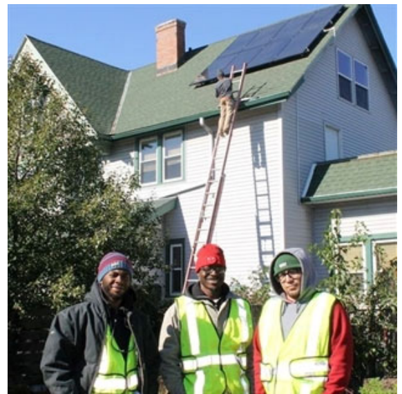
Rooftop solar installation
