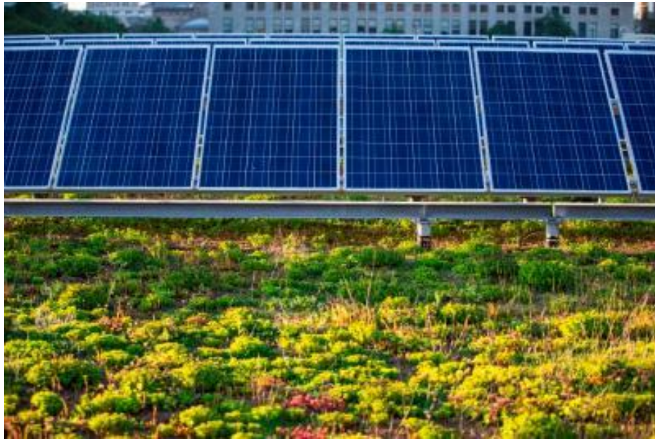
Solar panels on the Milwaukee Central Library roof
