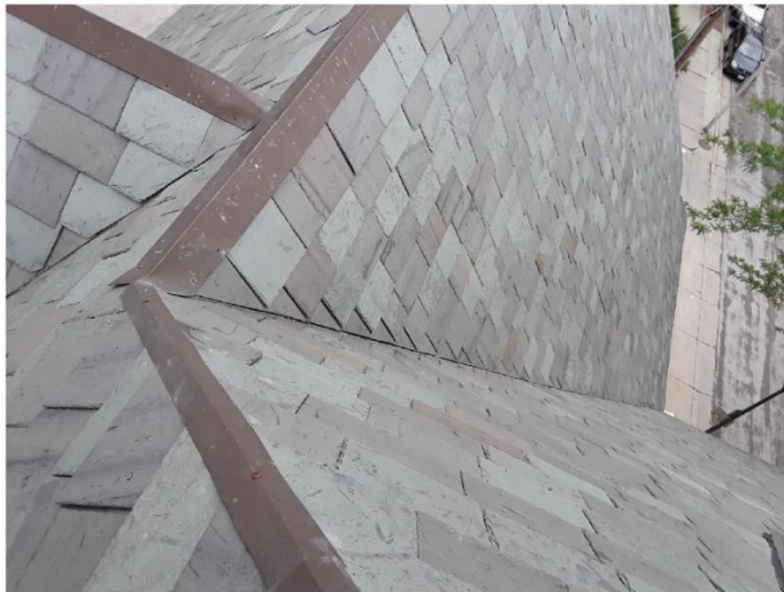
The current slate was installed about 10 years ago and the roof has failed. It is a mix of grey and green slate and not appropriate for this building.
