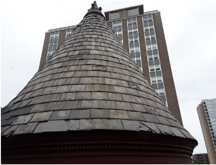
The new slate roof will match the original 1880 roof which is still on the tower. Buckingham Virginia slate will be used.
