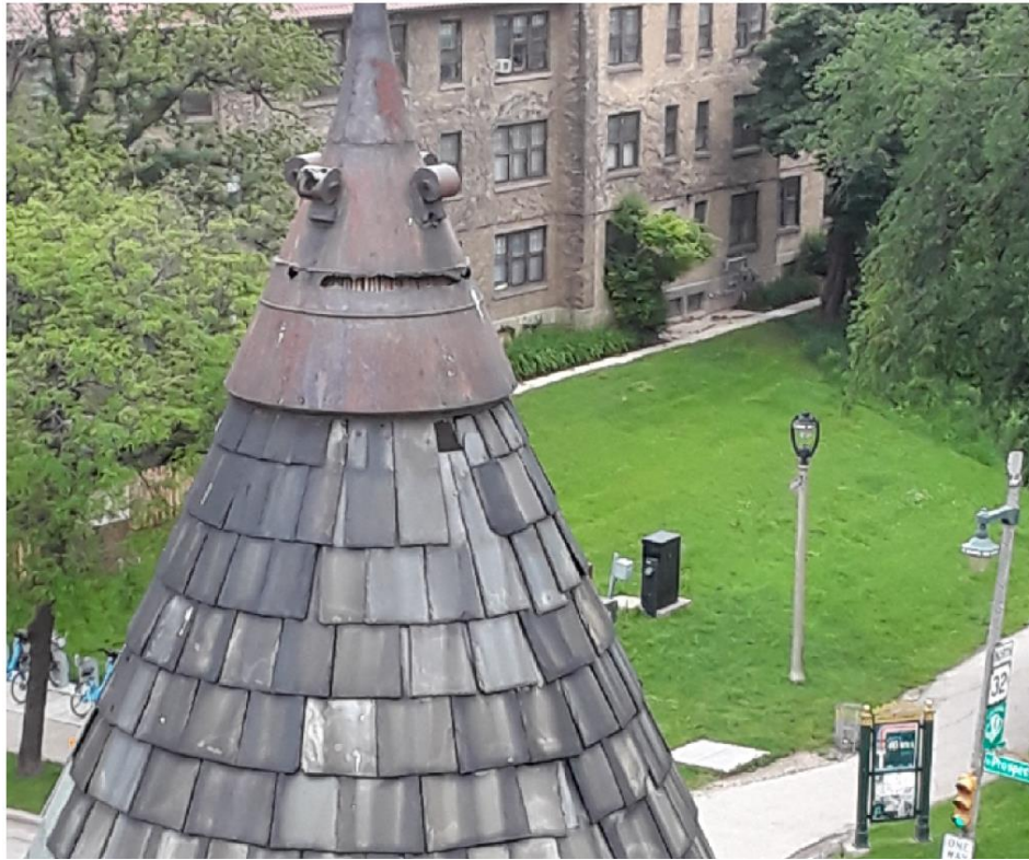
Damaged finial will be replicated exactly in new cuprous material.
