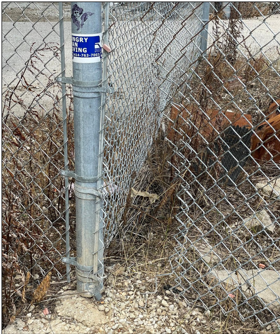
FIGURE 13.—Example of Perimeter Fence Compromise.
