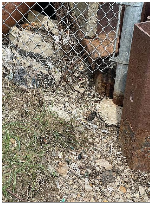
FIGURE C-5.—Example of Fencing in Poor Condition.
