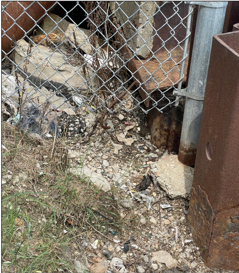
FIGURE 12.—Example of Fencing in Poor Condition.
