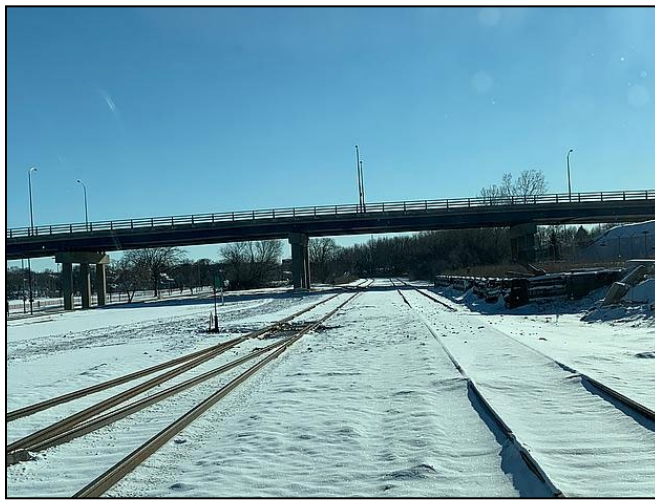
FIGURE C-19.—View of Rail Spur Demarcation Points Looking South on Access Road Illustrating no Rail Gates.
