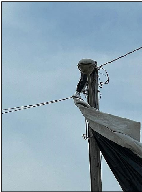
FIGURE C-9.—Example of Salt Coverage Tarps Wrapped around Electrical Service Line.
