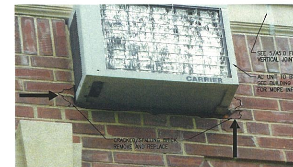
16 CRACKING/SPALLING BRICK AT A.C. UNITS, TYP. SCALE: N.T.S.
