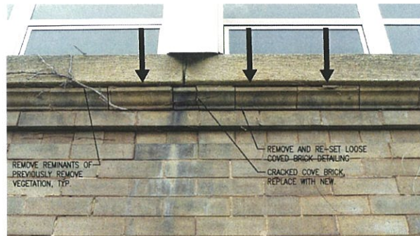
3 LOOSE AND CRACKING COVERED BRICK, TYP. SCALE: N.T.S.
