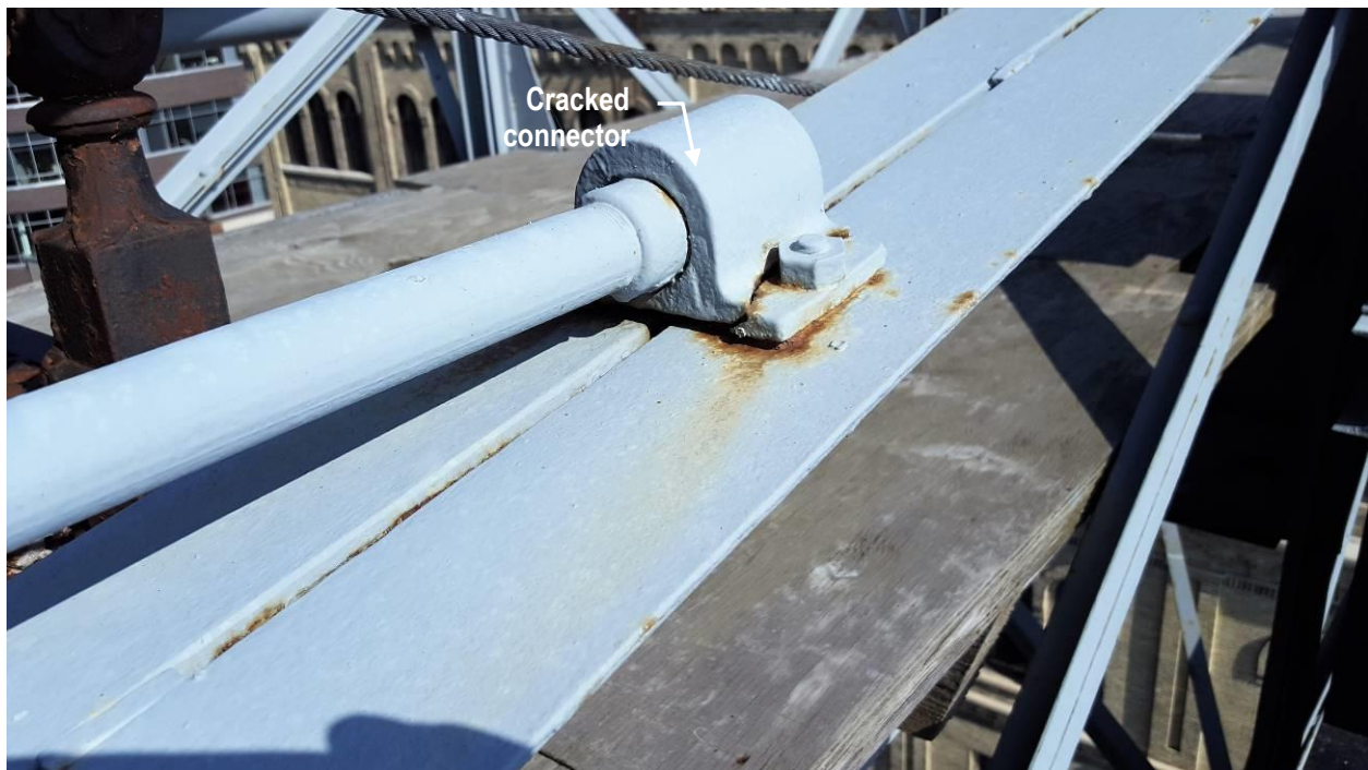
P16 Pabst sign bridge with cracked steel connector at guard rail (east truss).
