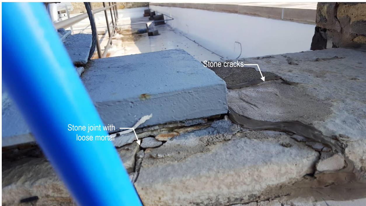
P18 Cracked and loose stone joints Pabst sign bridge (north support end).
