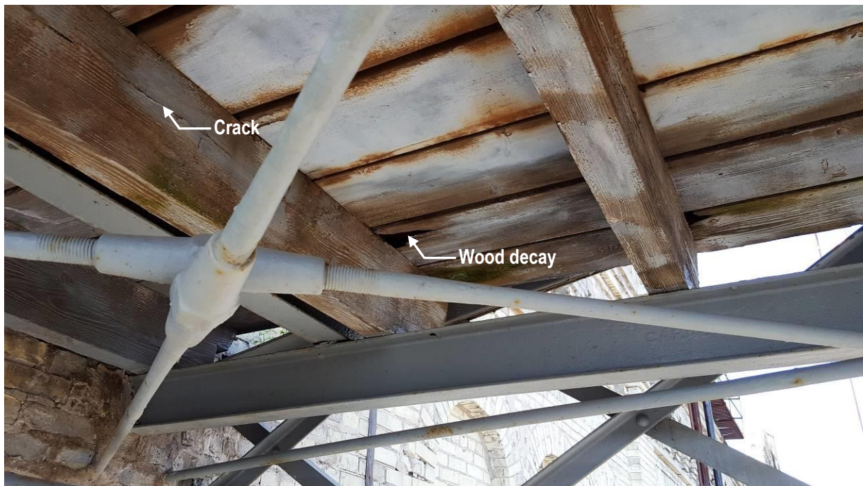
P6 Pabst sign bridge with cracked wood joist decay in wood decking
