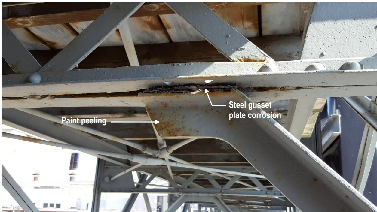
P9 Pabst sign bridge with corrosion at interior transverse open web steel joist support.
