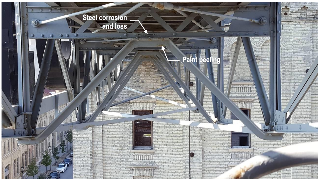
P10 Pabst sign bridge with steel corrosion and loss at interior transverse open web steel joist support
