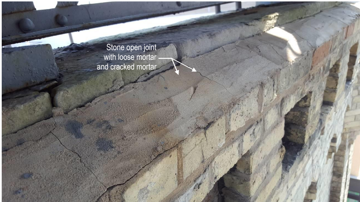
P19 Cracked and loose mortar grouts (north support end).
