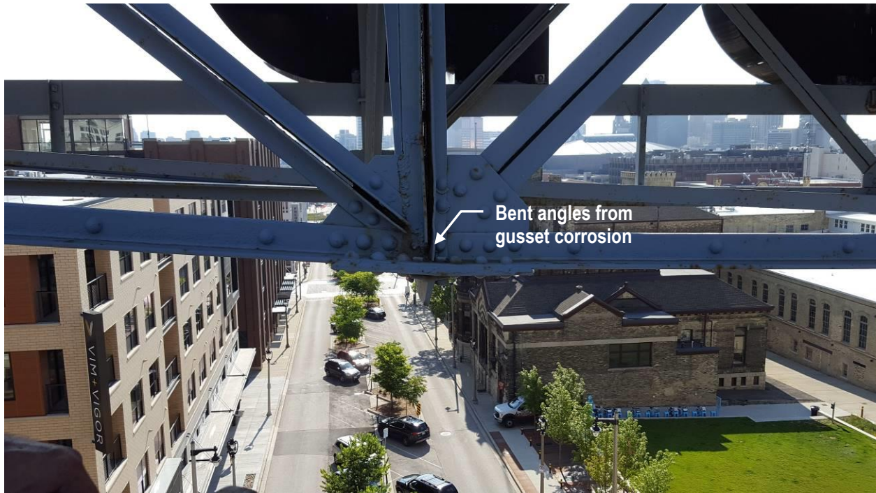
P13 Pabst sign bridge with bent steel angles and section loss from corrosion at panel point (east truss).
