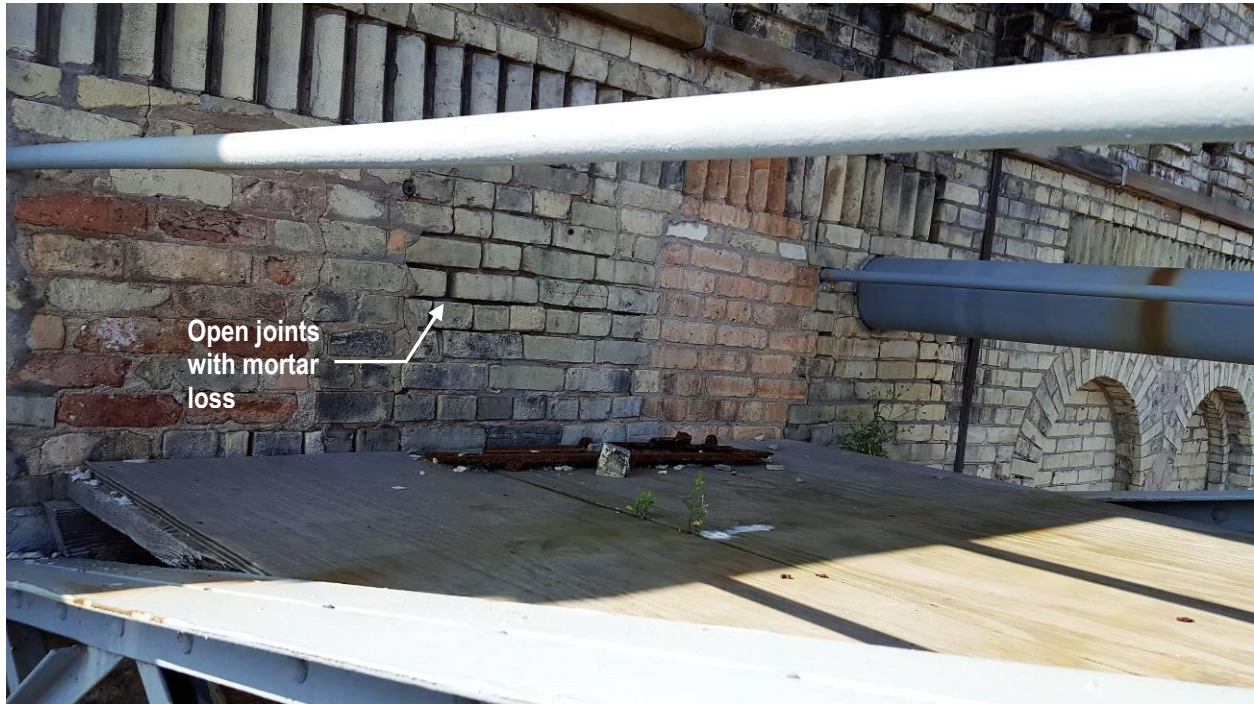
P17 Open joints with mortar loss at Pabst sign bridge south support end.
