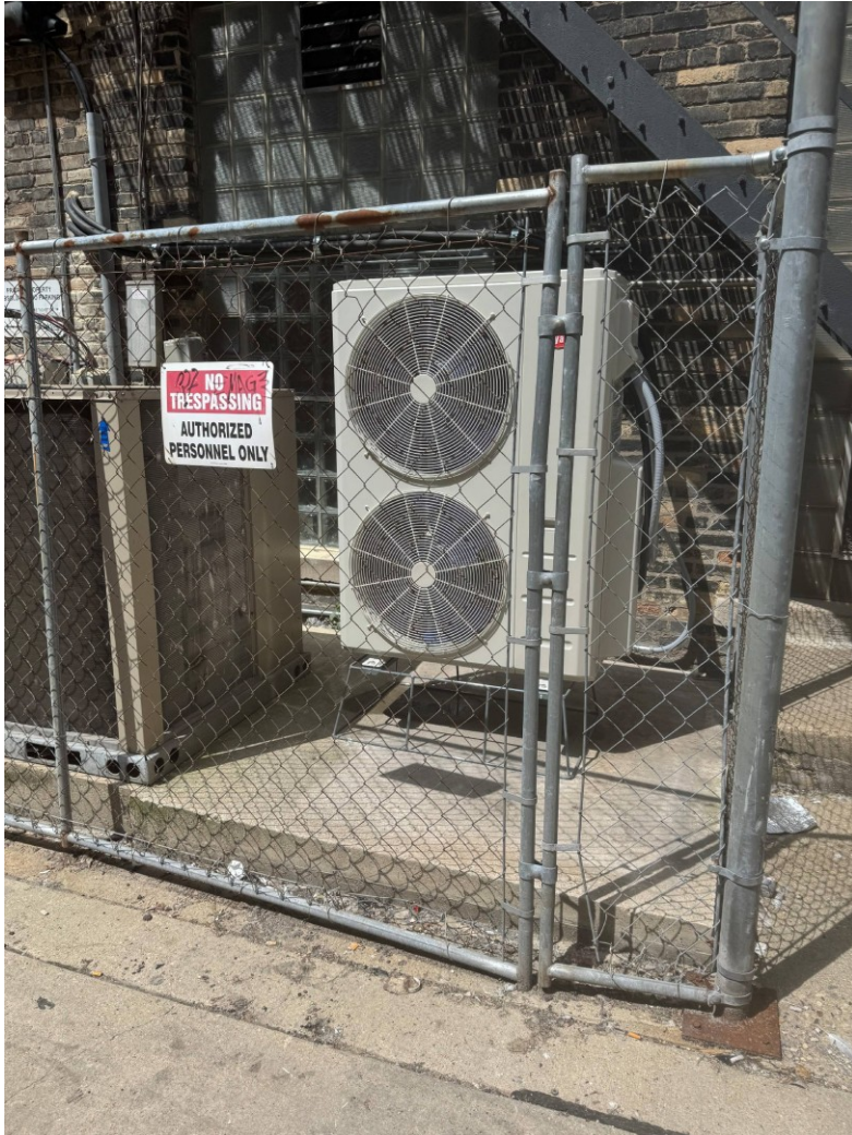
Air handler to be replaced
