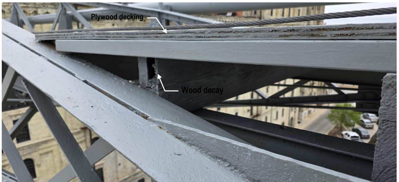
P8 Pabst sign bridge with end rotted wood joist (east elevation).
