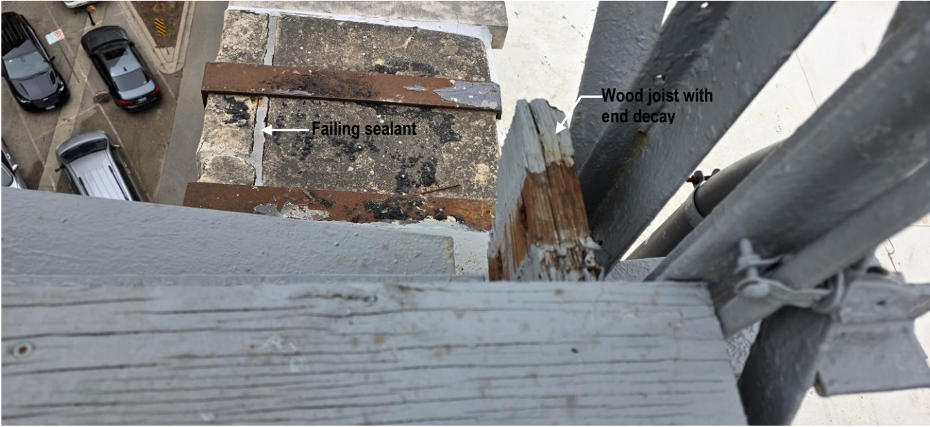
P9 Pabst sign bridge with end rotted wood joist (west elevation).
