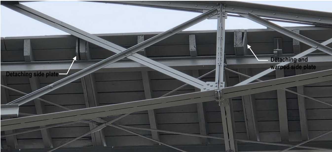
P10 Pabst sign bridge with detaching wood plates in wood joists.
