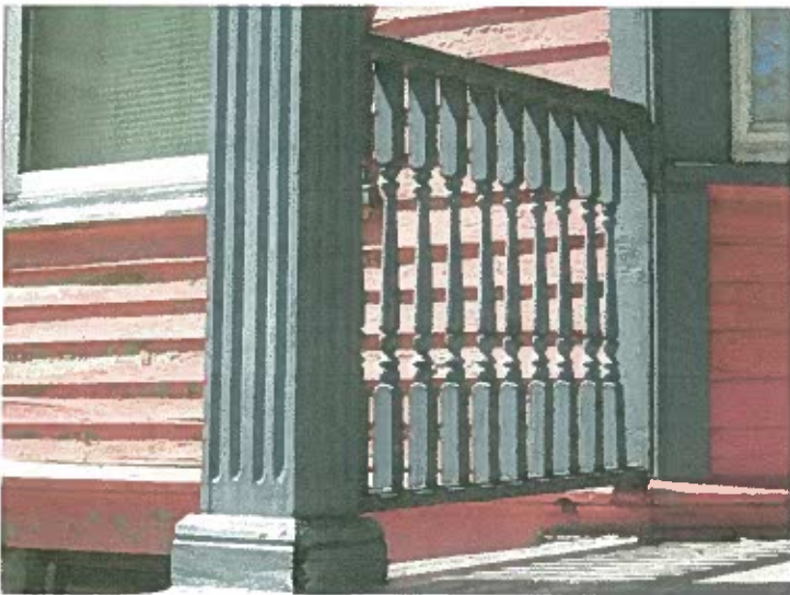
4. Front Porch south railing and column deterioration
