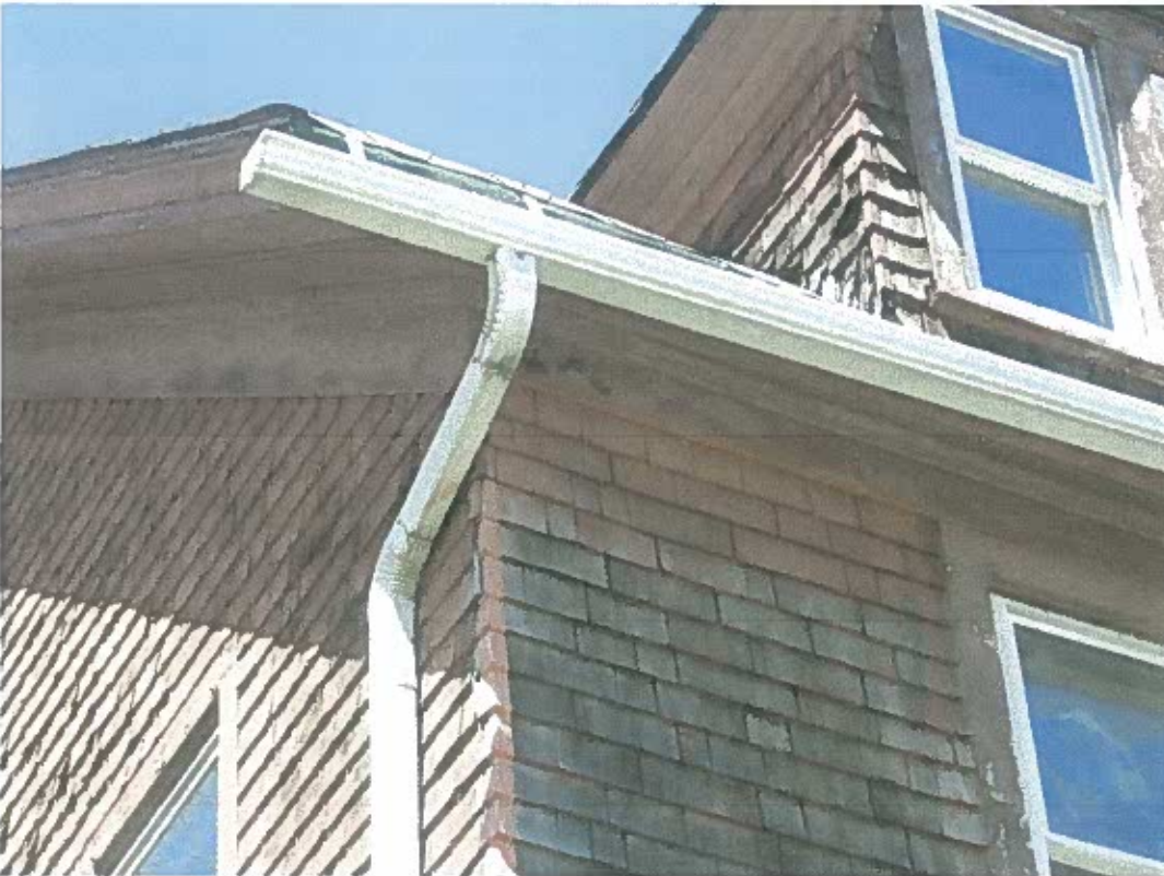
7. Second floor (South-East Elevation) cornice line connection showing new K-Style gutters and shingle deterioration
