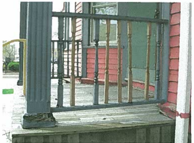
5. Front Porch north railing and column deterioration
