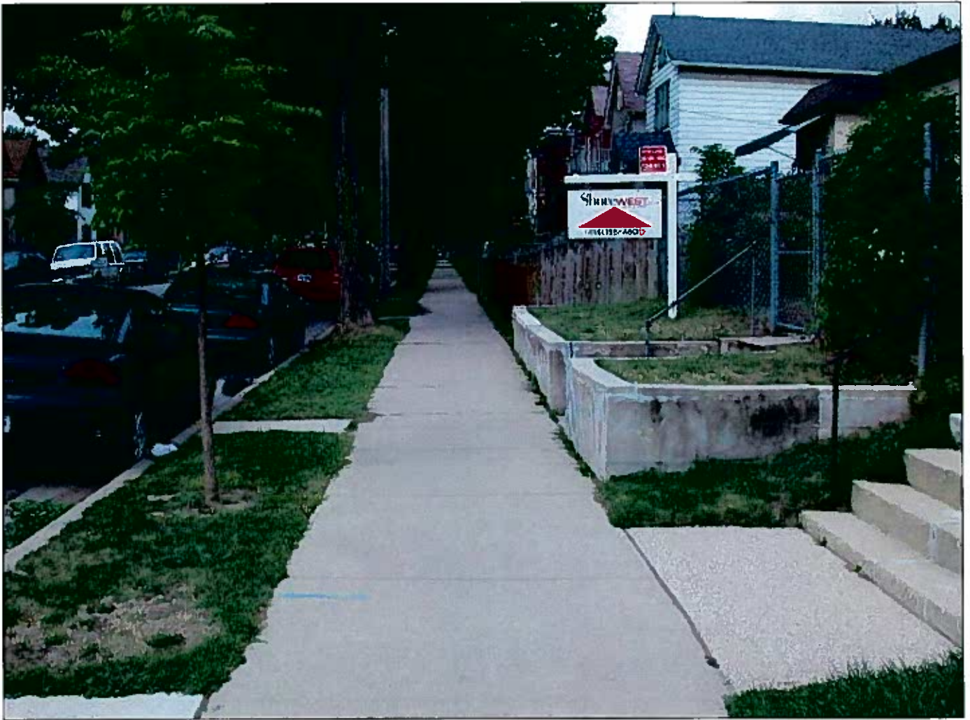
1222 W. Washington CCF 080513 09/15/08 Looking west on W. Washington St. at the Retaining wall
