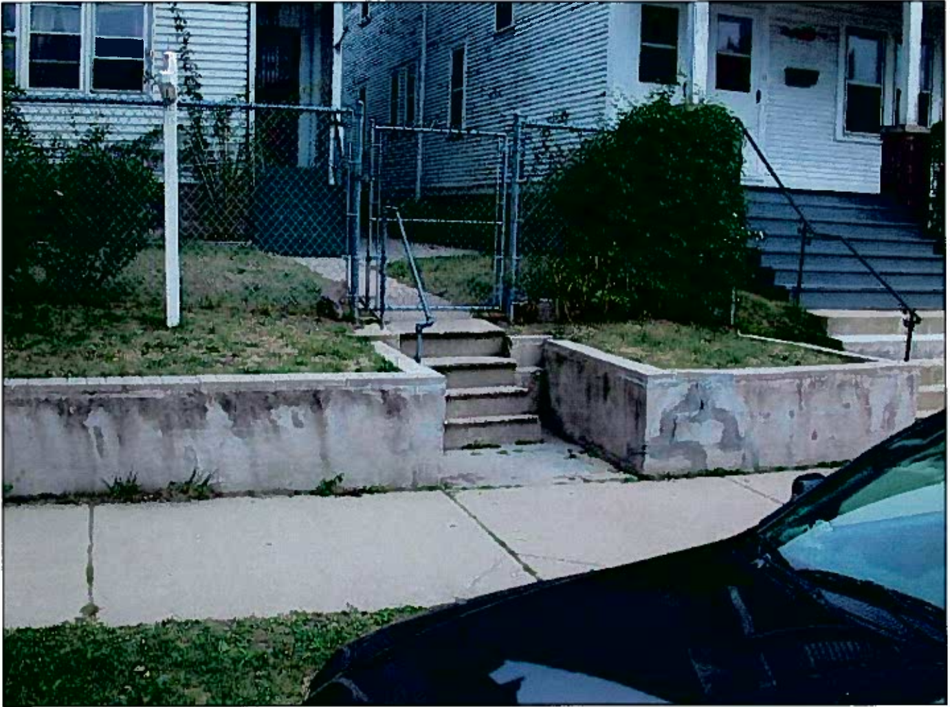
1222 W. Washington CCF 080513 09/15/08 Looking north on W. Washington St. at the retaining wall and steps
