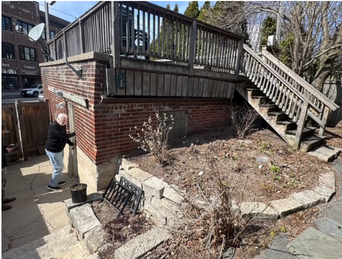
Existing garage deck to be rebuilt in-kind with molded top and bottom rails and baluster design provided above
