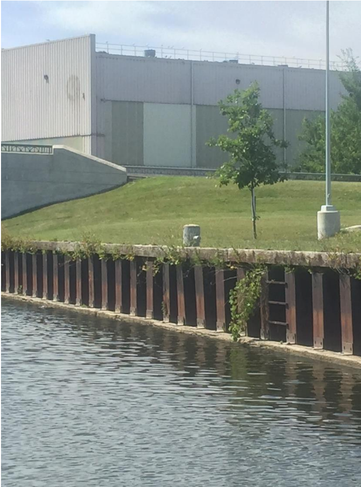
Example of existing water edge condition where legal boundary is likely corresponding to a physical element such as the sheet pile seawall.
