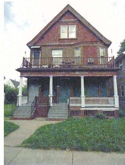
This is one of four boarded up properties on the block.
