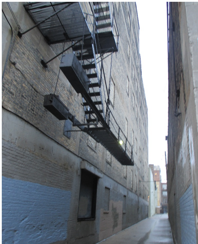
Photo 24 - 12.23.14: North façade of main building and vacated alley between main building and storage building
