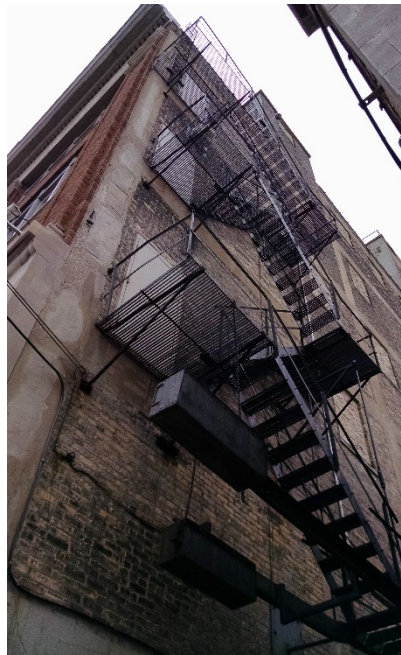
Photo 14 - 5.12.15: Fire escape stairs on northeast corner of main building
