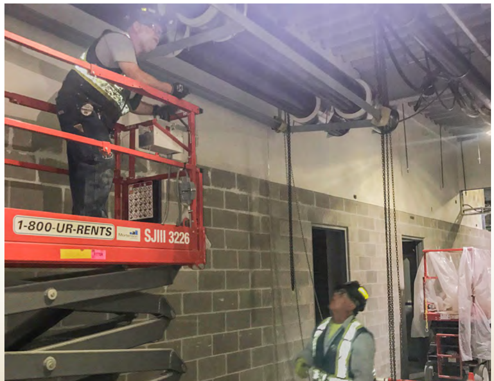
Right: PL Freeman Co. employees working on HVAC piping for the arena.
