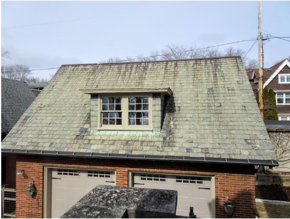
Rusted tin flashing to be replaced with new 20 ounce ridge.
