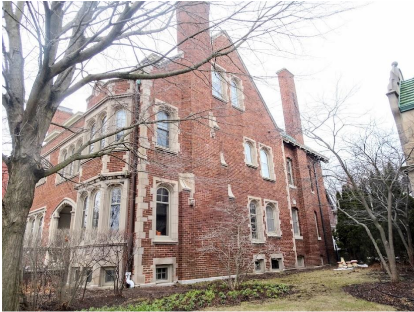
North elevation gutter and downspout to be replaced
