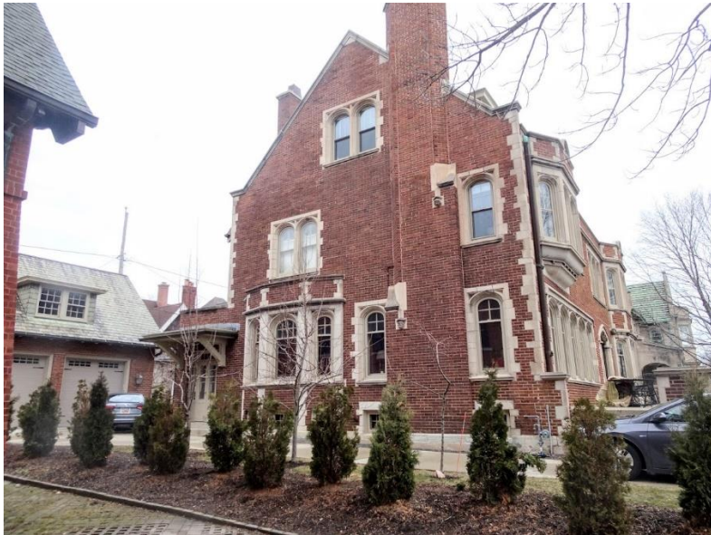
SE corner downspout to be replaced
