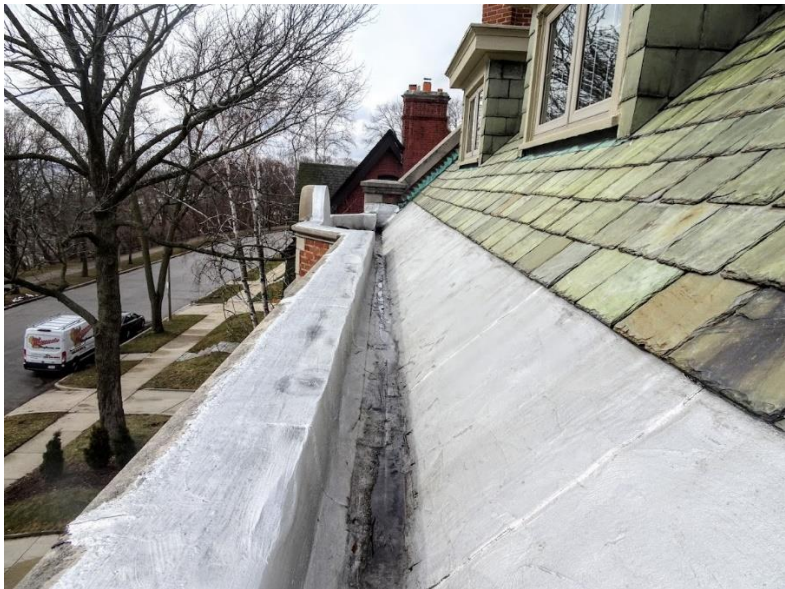
Roof trough to be patched
