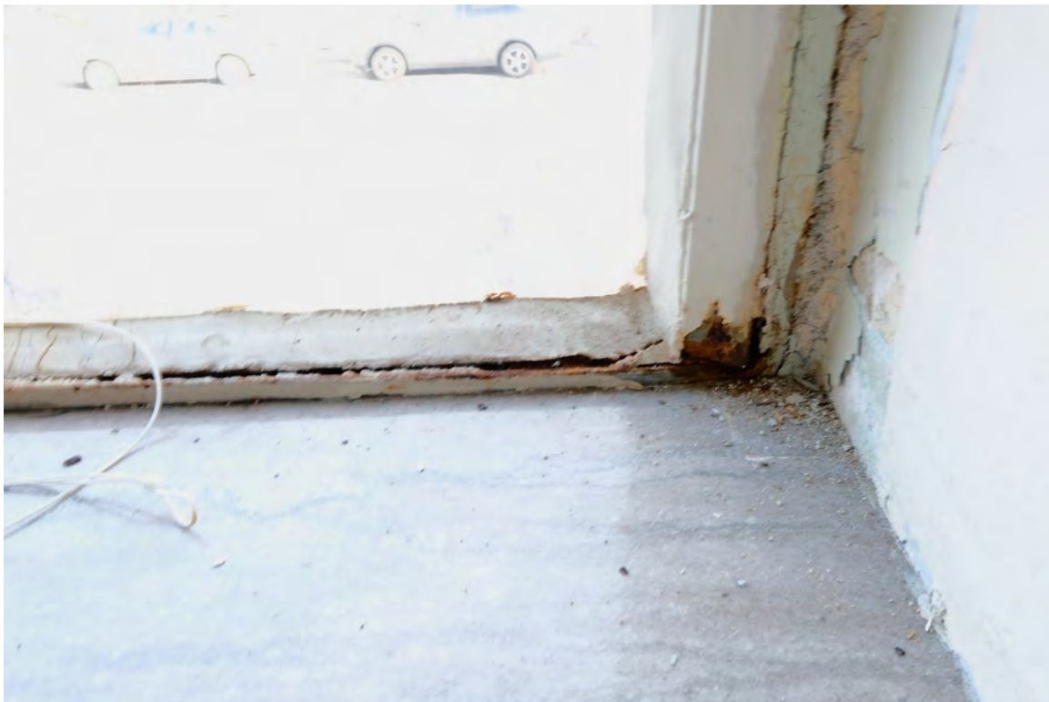
IMAGE 6: Typical corrosion location at the frame corners. Also note expansion cracks at frame and cracked sealant. Preserve, LLC 2021.
