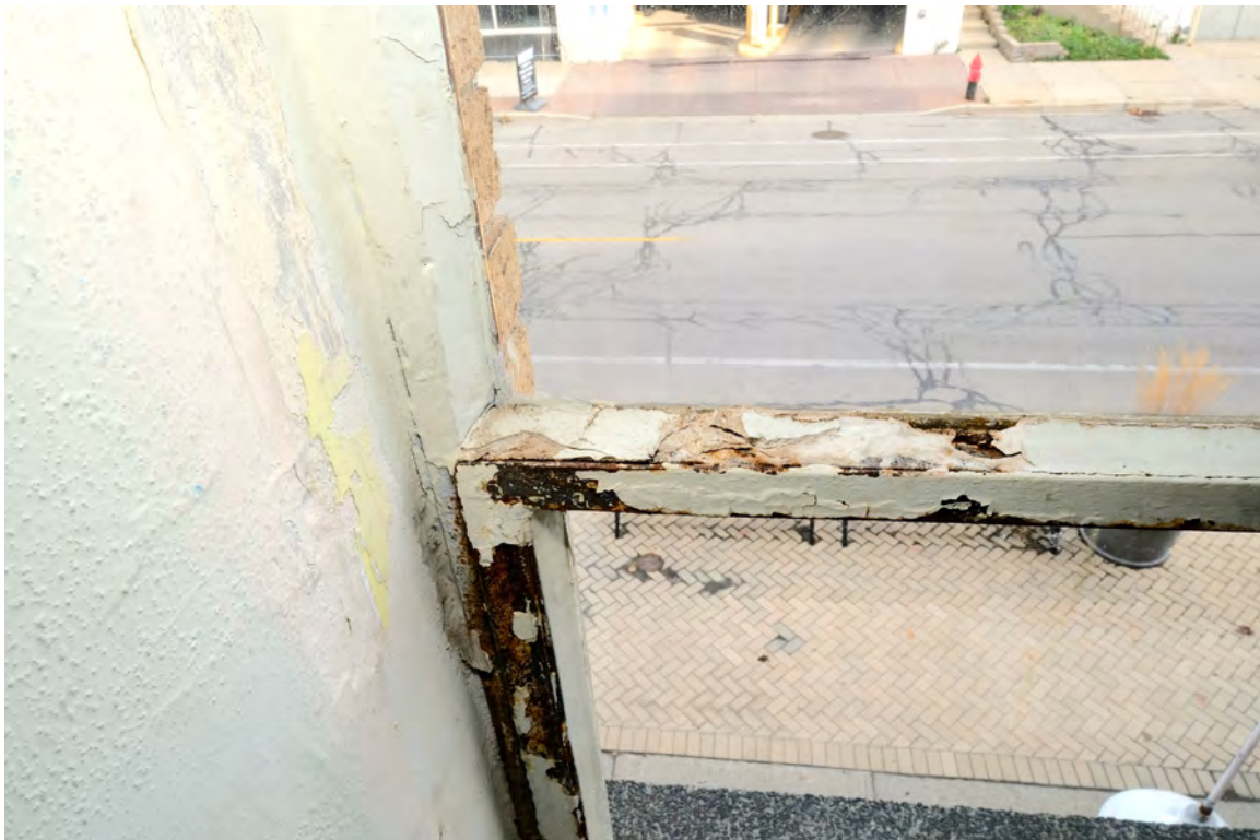
IMAGE 12: View of corrosion at ventilator frame. Seized frames, corrosion, paint, and missing hardware prevent window units from operating. Preserve, LLC 2021.
