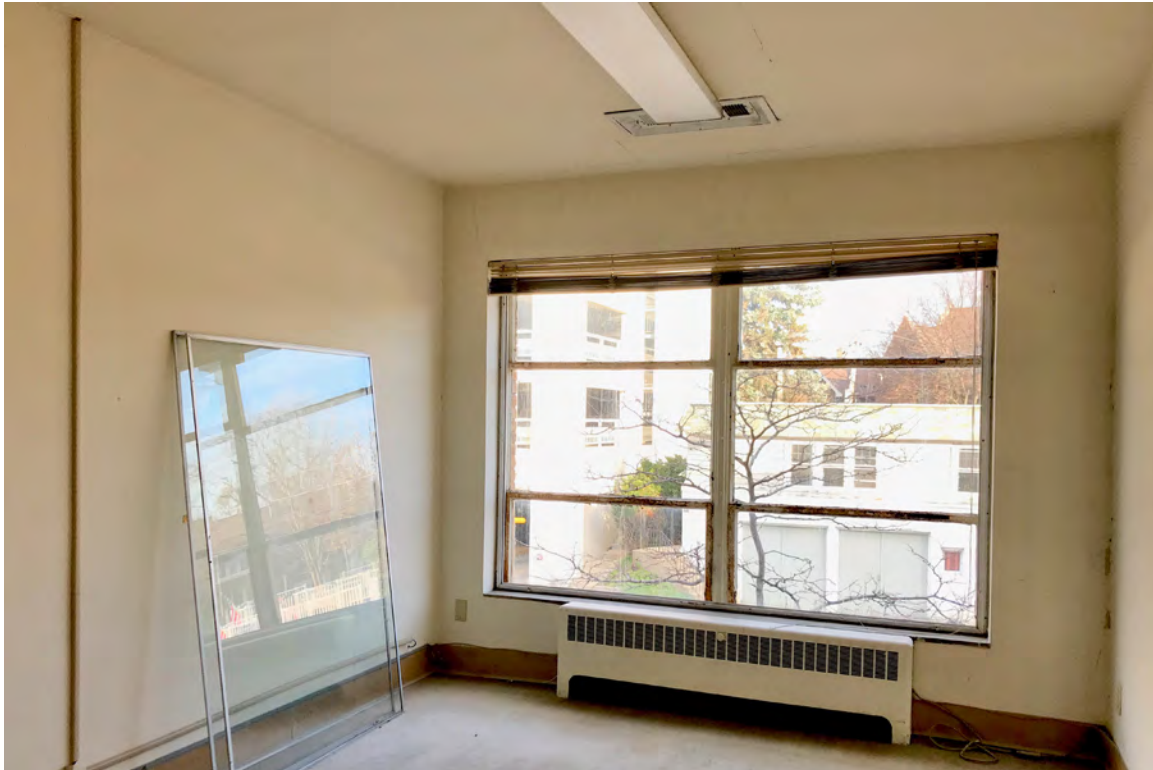
IMAGE 19: View of typical window unit. Corrosion is heaviest at the operable sash. Preserve, LLC 2021.
