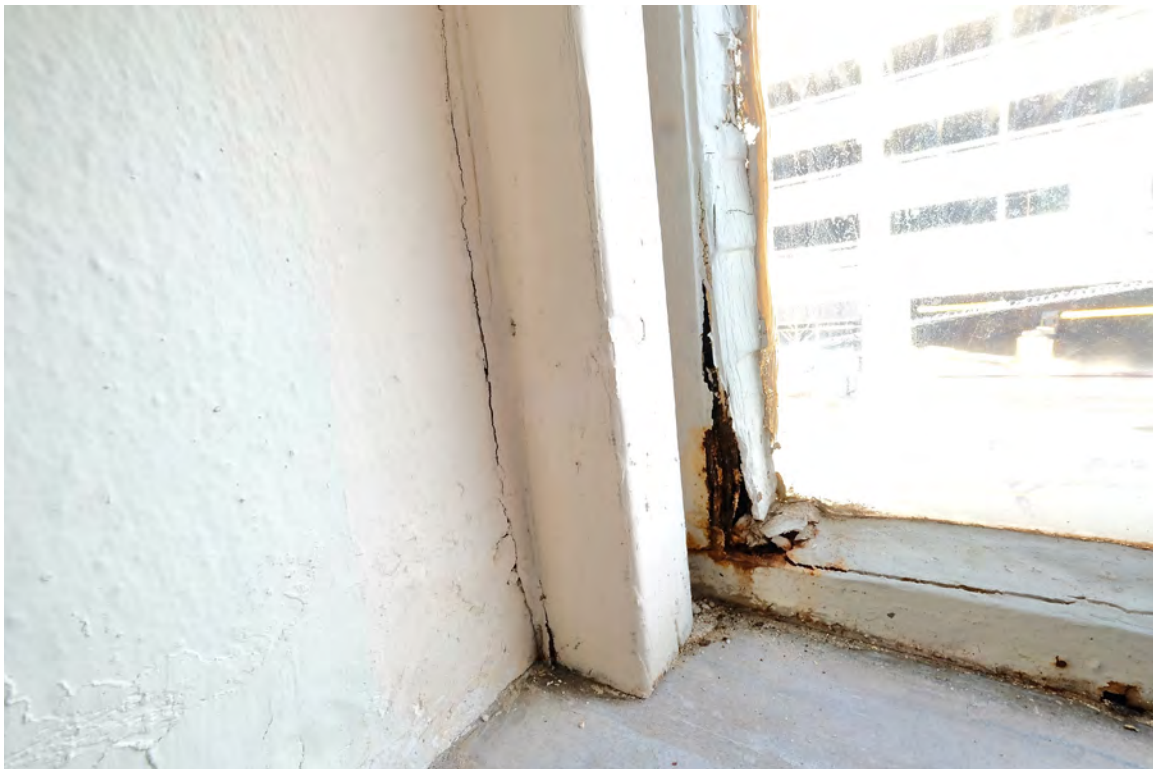
IMAGE 10: Corrosion typical at frame corners. Select units have interior storms installed. Preserve, LLC 2021.
