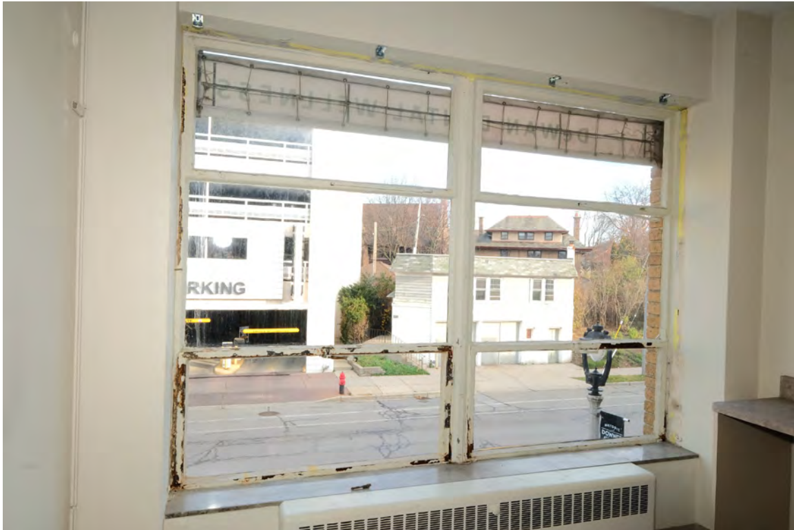
IMAGE 11: Interior view of a typical second-floor unit with typical corrosion throughout. Preserve, LLC 2021.
