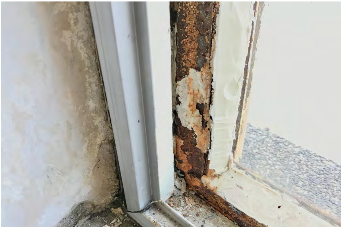
IMAGE 18: View of heavily deteriorated and corroded corner of window frame. Preserve, LLC 2021.
