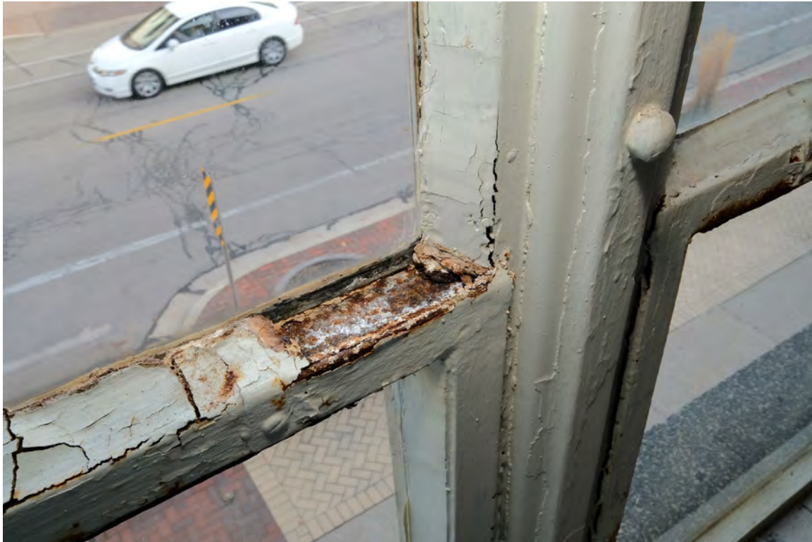
IMAGE 9: Corrosion typical at mullions. Preserve, LLC 2021.
