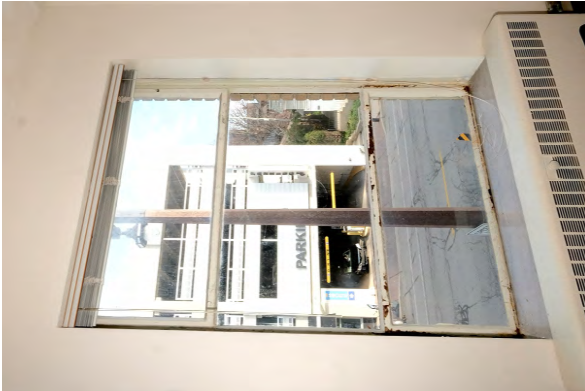
IMAGE 5: Corrosion is typical on the interior side of units. Window units have been painted closed. Preserve, LLC 2021.
