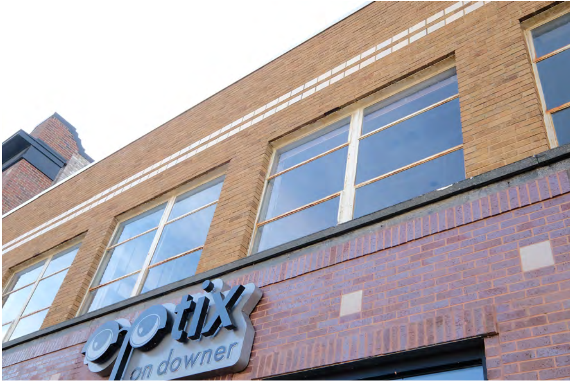
IMAGE 3: Typical east elevation second floor windows. Corrosion is evident throughout. Preserve, LLC 2021.
