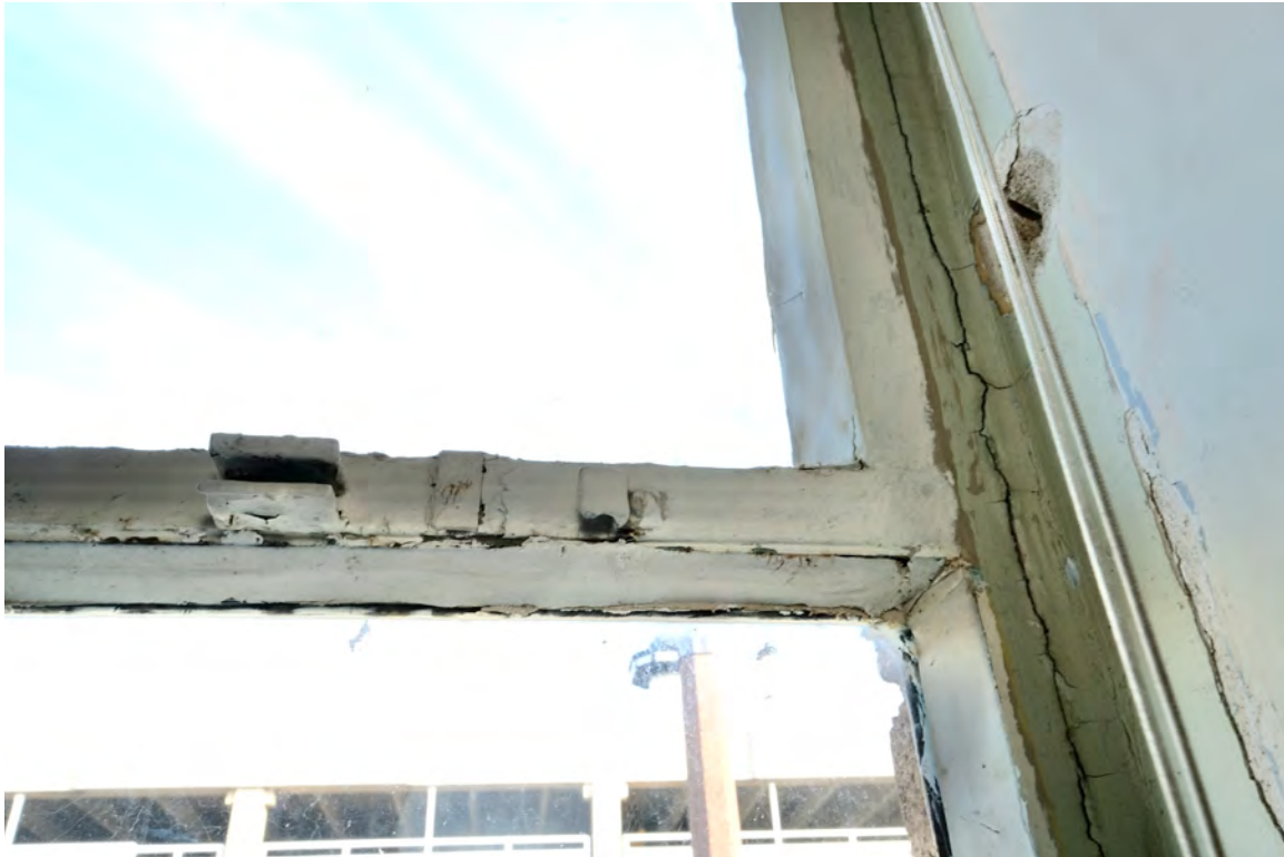
IMAGE 7: View of operable sash. Sashes are painted closed and cranks and hardware has been removed at spot locations throughout. Preserve, LLC 2021.
