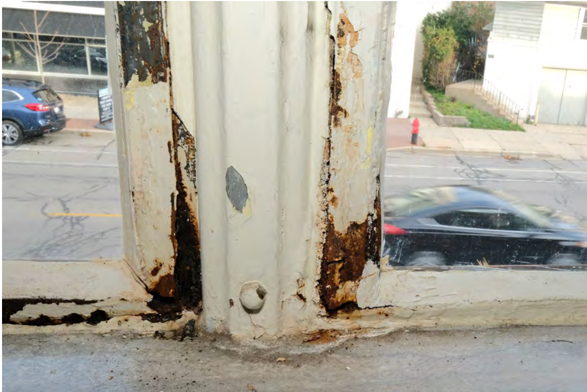
IMAGE 13: View of typical corrosion at window frame corners at center mullion. Preserve, LLC 2021.
