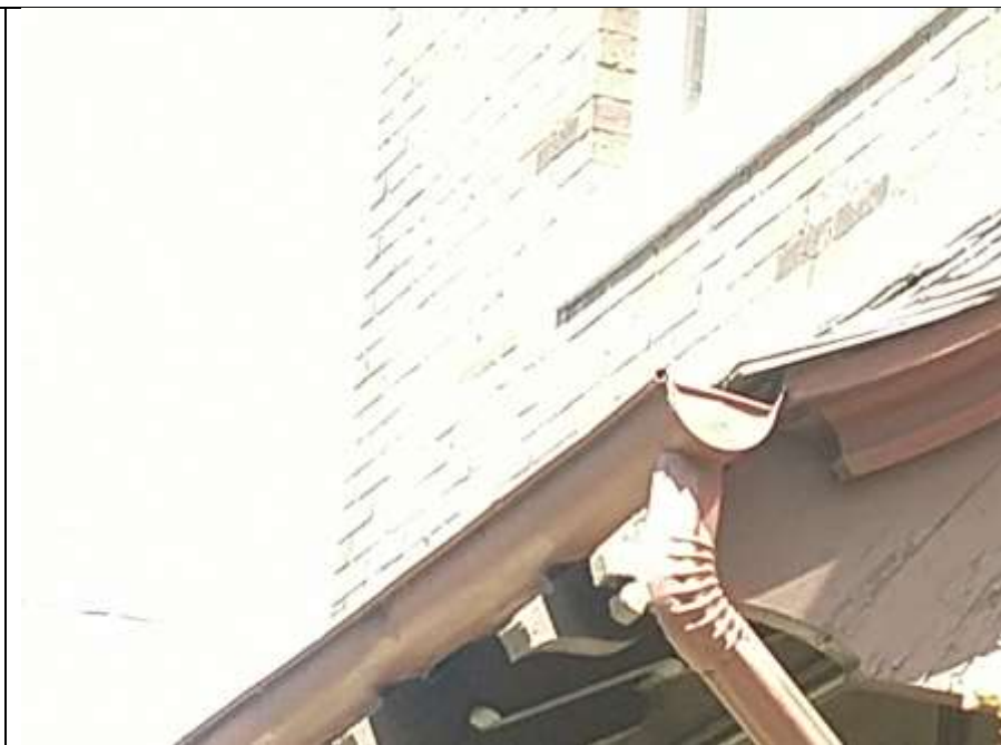
Type of gutter to be removed and replaced with replicas of gutters at left.
