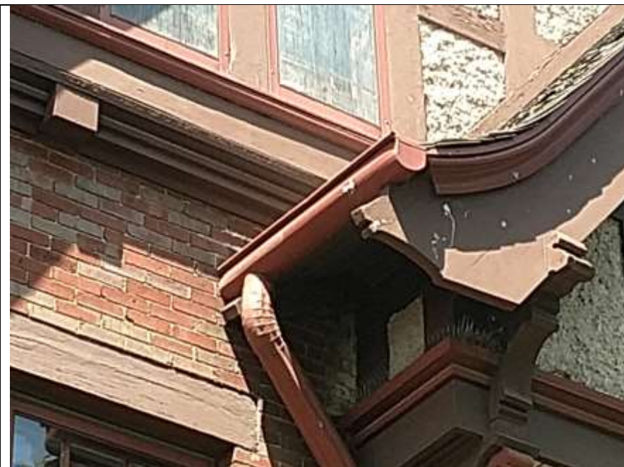
Original high back gutter type to be replicated where needed.
