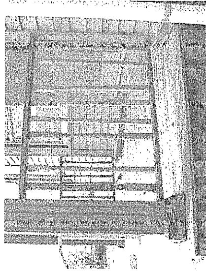
5. Front Porch north railing and column deterioration
