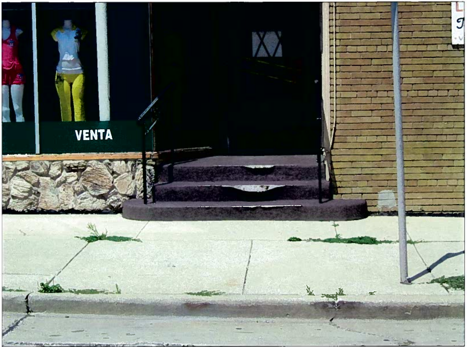
2972-74 South 13th Street CCF 080297 8/1/08 Looking North on West Manitoba Street at the concrete step with handrail and carpet
