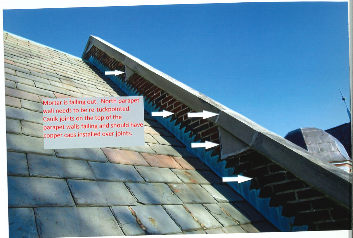
Caulking on parapet cracking and letting water into the wall below. Counter flashing coming loose from
