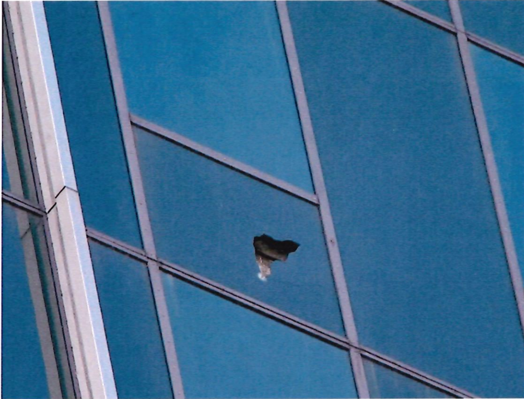
A broken window can be seen in one of the upper windows of the Chase Tower at 111 E. Wisconsin Ave in downtown Milwaukee on Thursday, April 14, 2022. Glass reportedly fell from the 22-story building to the pavement below, prompting police to close sidewalks. Angela Peterson/Milwaukee Journal Sentinel
