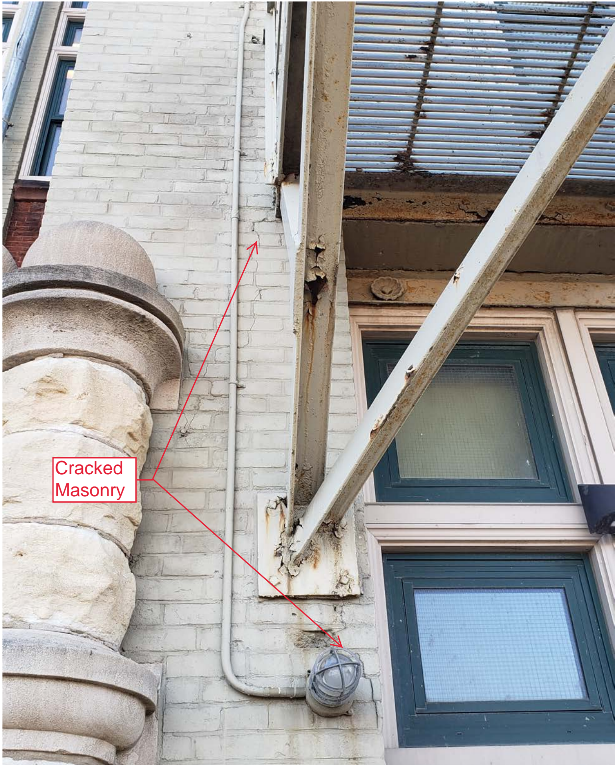
Figure 6 Cracking Masonry at and Around Fire Escape Support Brackets
