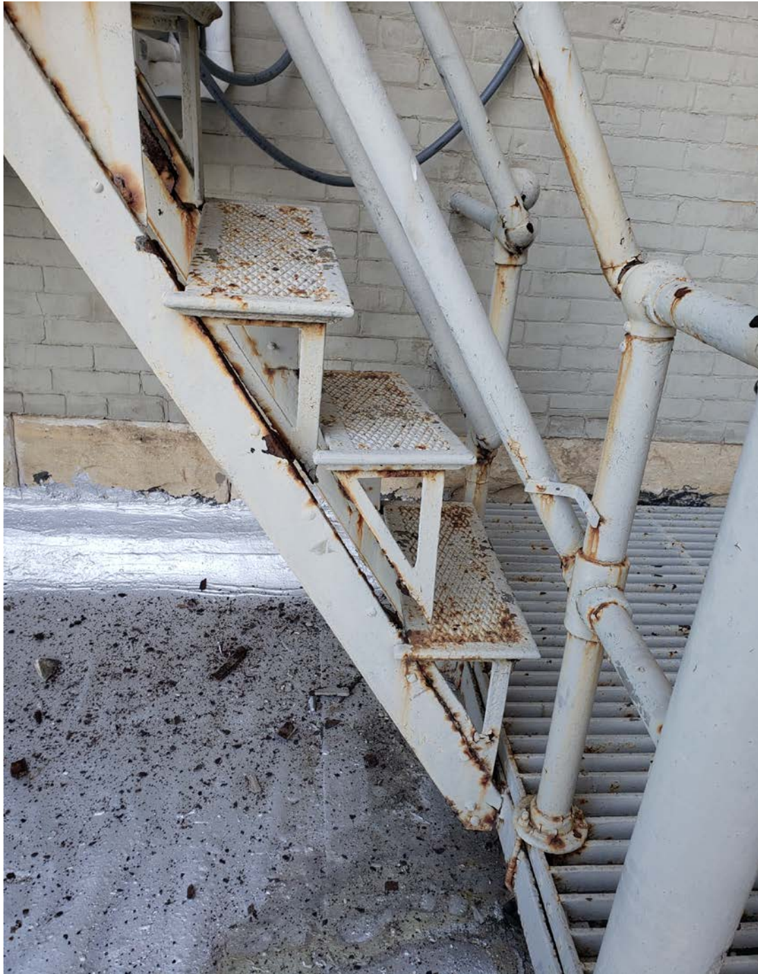
Figure 7 Failed Tread Bracket Connection
