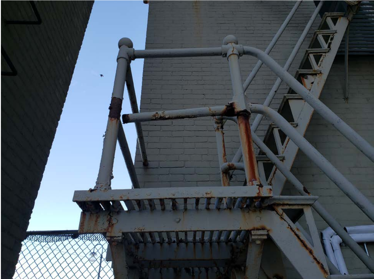
Figure 7 Broken and/or Missing Railing Connection Brackets
