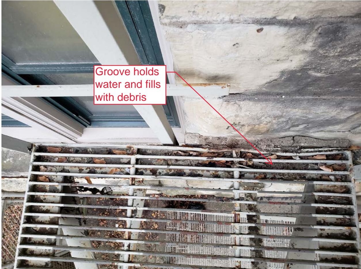
Figure 5 Enclosed Grooves of Bar Grating Trap Water and Debris Which Accelerate Corrosion
