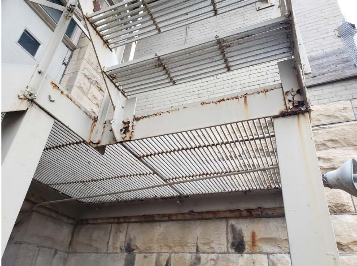
Figure 4 Common corrosion found on FE#1 and FE#2
