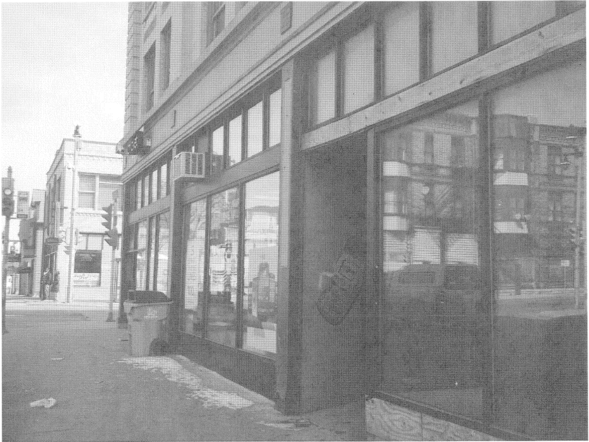
Image 35 - Date: 01-16-2014 – North Elevation (Storefront Missing Aluminum Trim)
