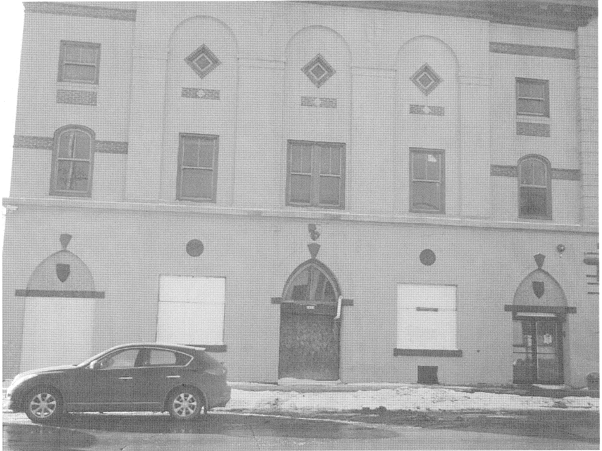
Image 41 - Date: 01-16-2014 – East Elevation (Windows & Doors Boarded Up)
