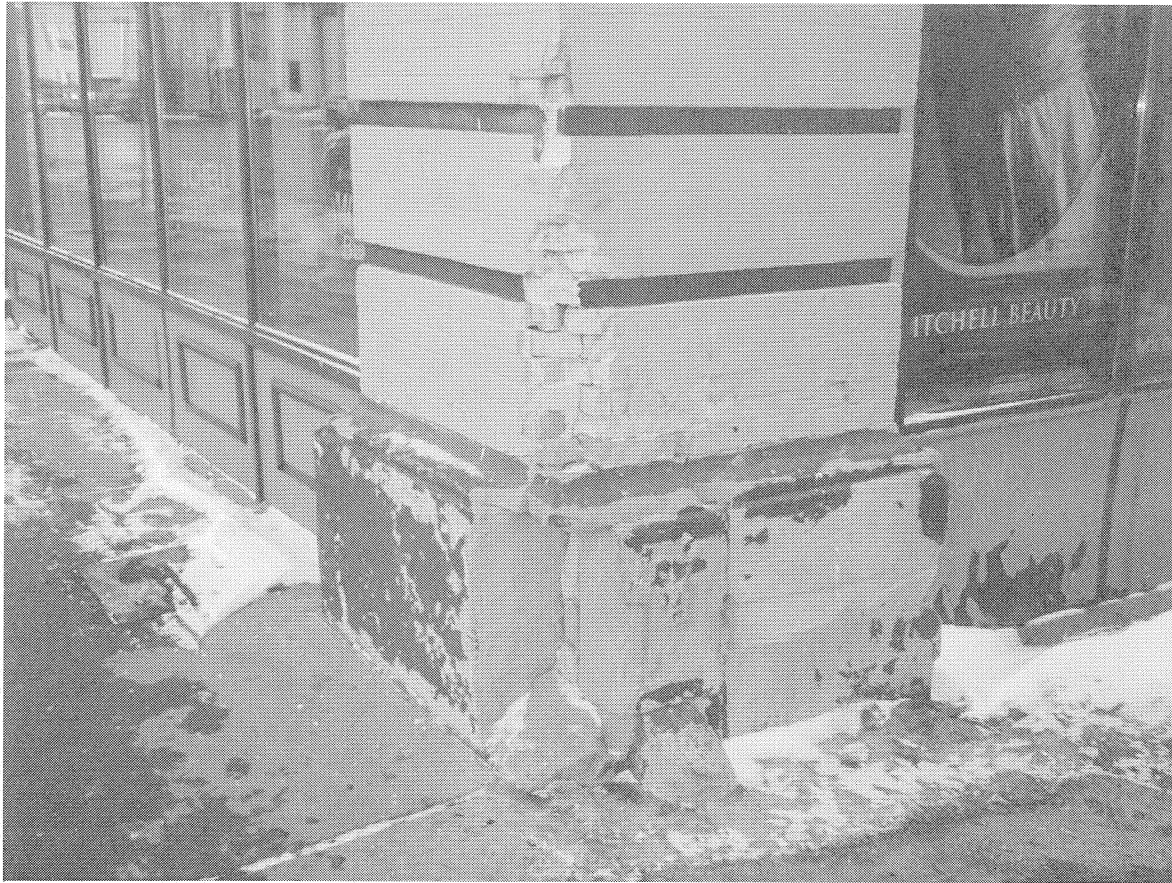
Image 29 - Date: 01-16-2014 - Damaged Northwest Corner and Missing Trim Under Existing Storefront
