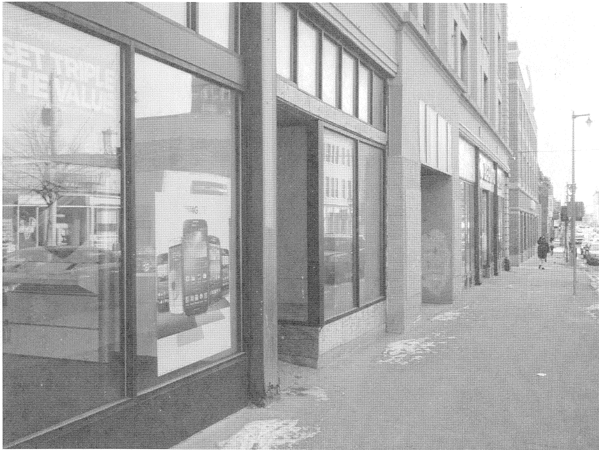
Image 34 - Date: 01-16-2014 – North Elevation (Storefront Missing Aluminum Trim)
