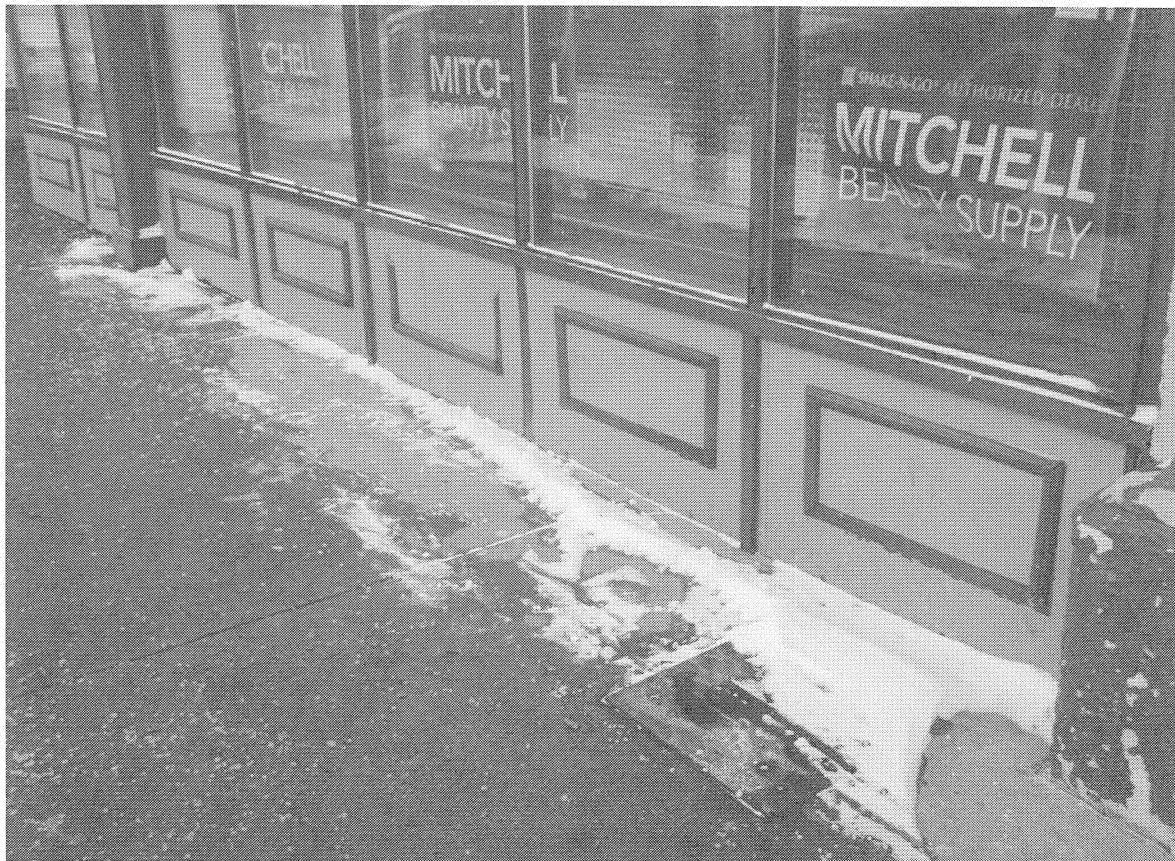
Image 30 - Date: 01-16-2014 - North Elevation (Damaged and Missing Trim Under Existing Storefront)
