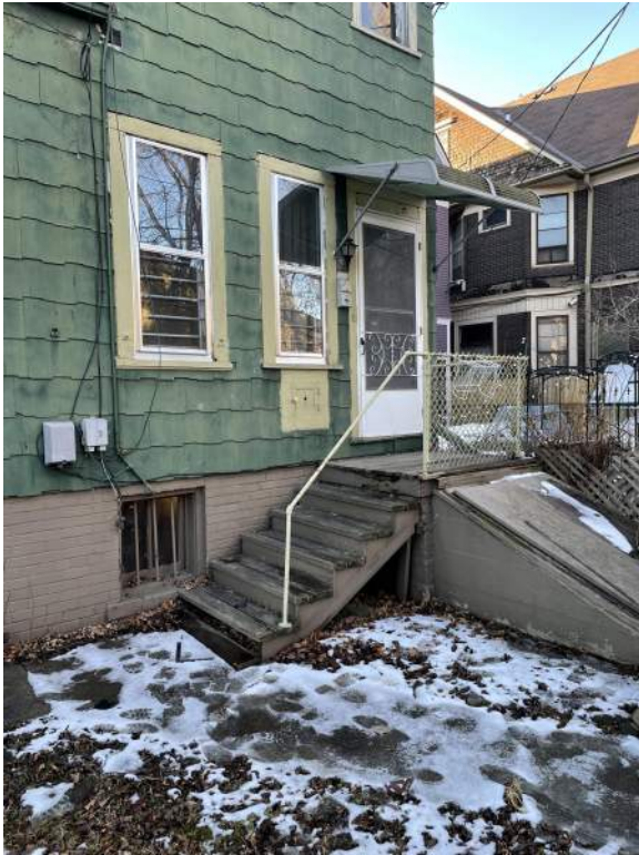
Photo 8 - Back Exterior Stairs Showing Deterioration
