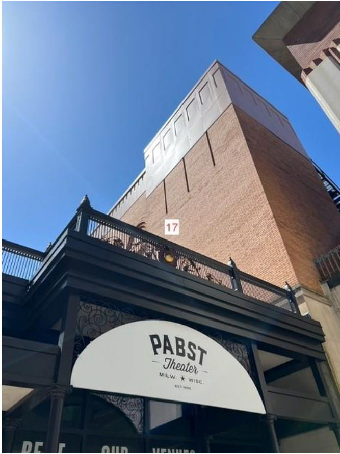
Areas of railing repair and re-gilding
