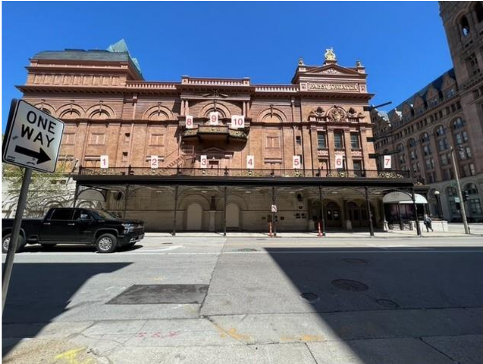
Areas of railing repair and re-gilding
