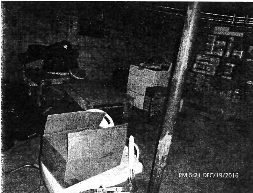
storage in mech room
