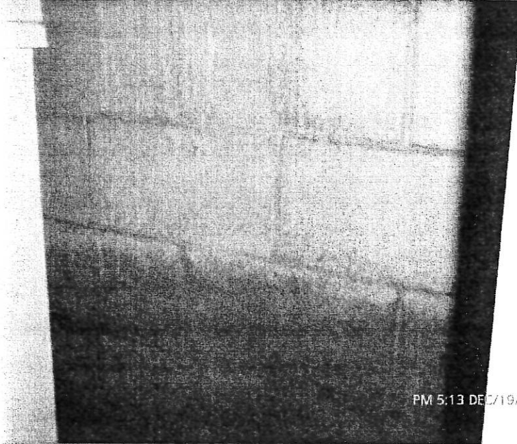
water lines in mech room
