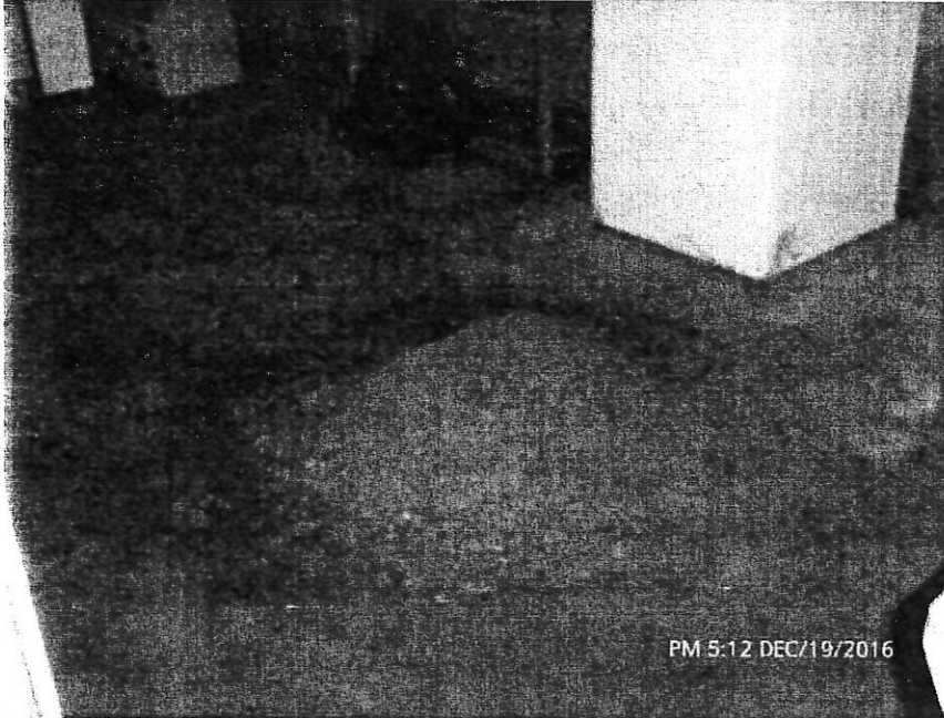
Floor drain, debris that came back up
