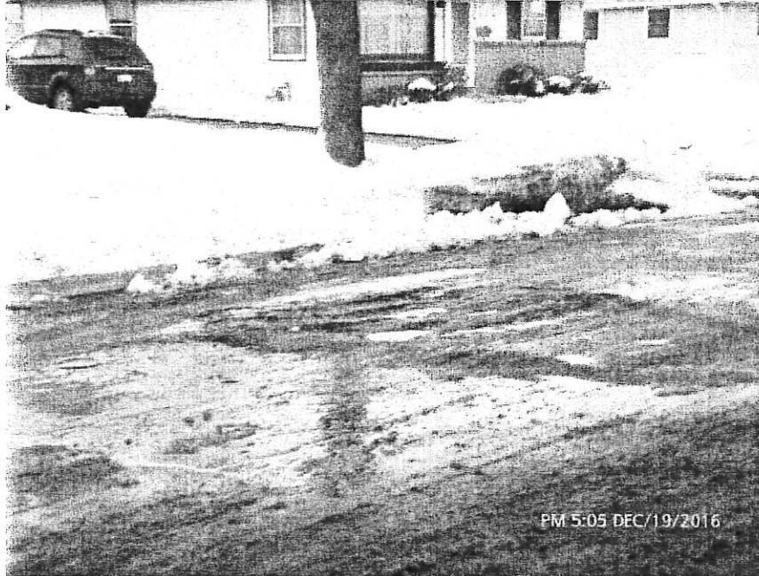
Sink Hole in front of home
