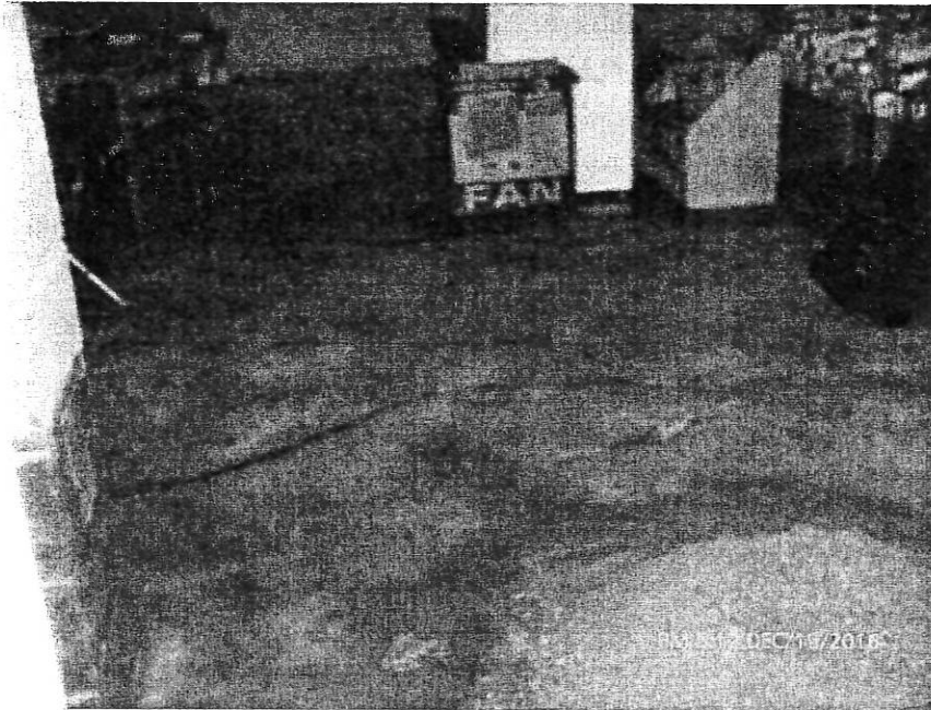
Floor drain, debris that came back up
