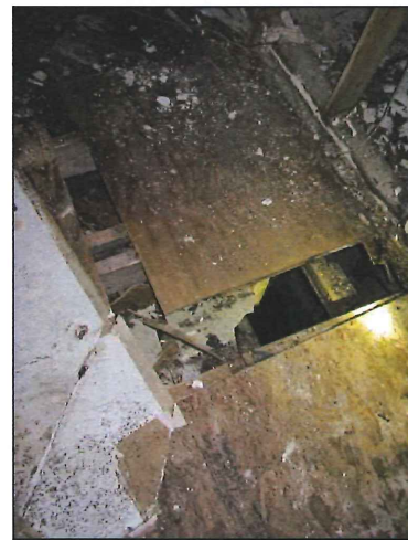
View of hole in front room floor
