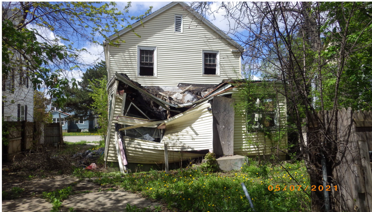
View southwest towards collapsed addition at the subject property.
