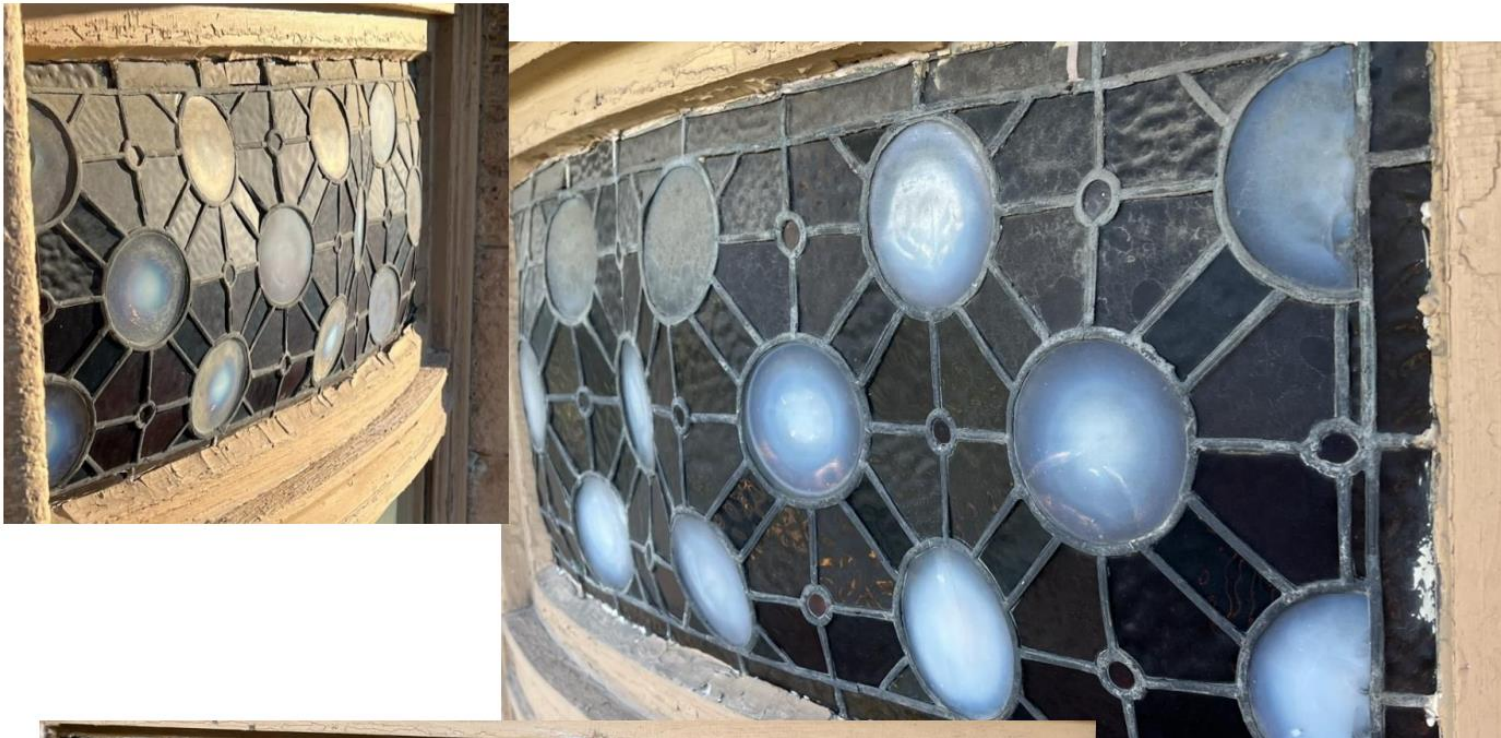
Typical damage, note outward bulge of glass
