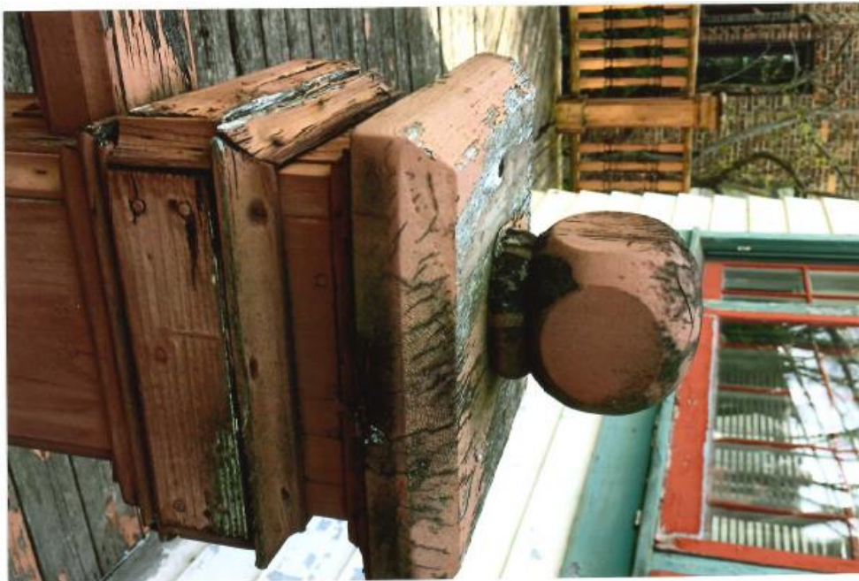
Existing finials to be replaced.
