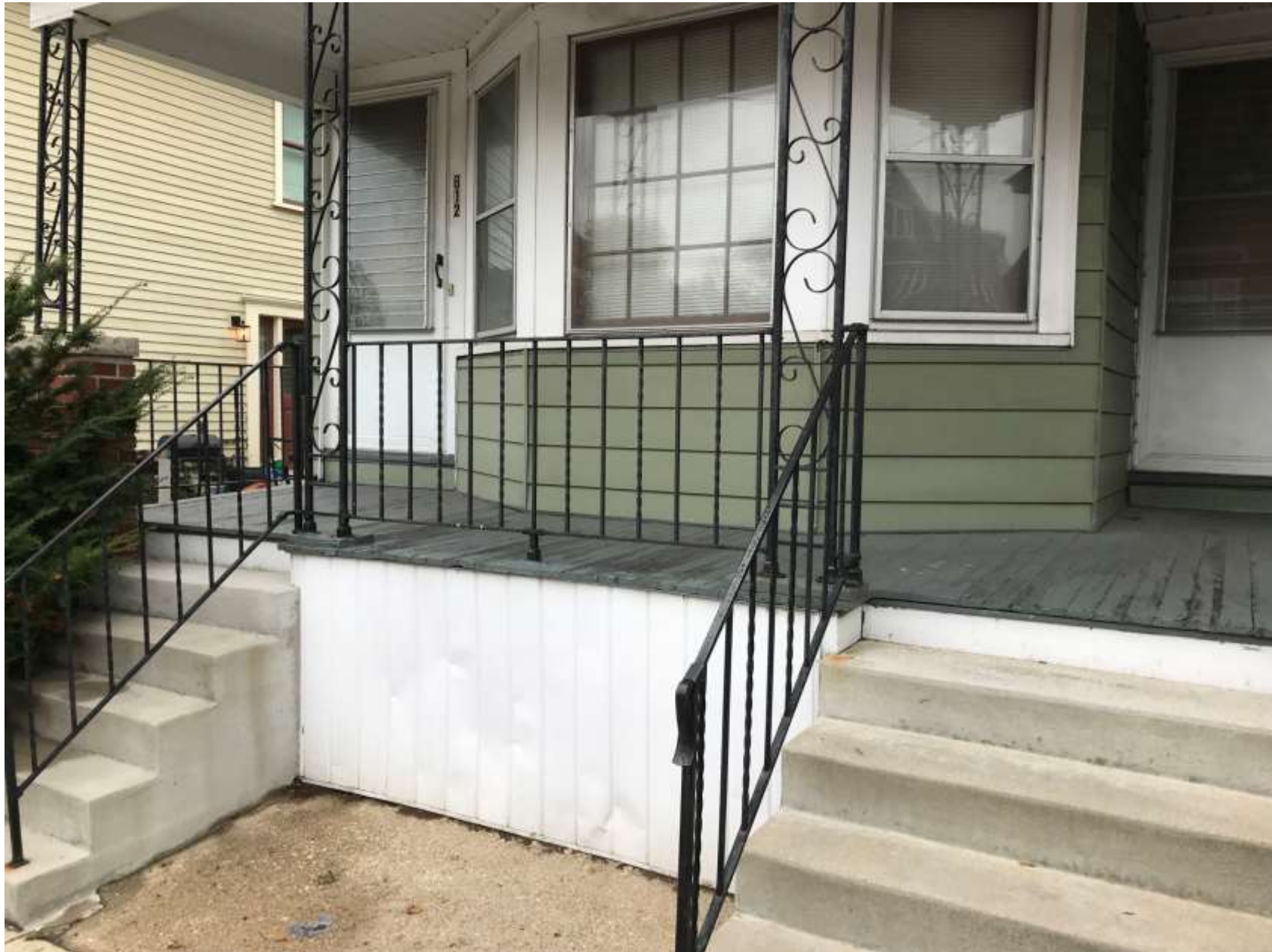
East end of porch is at left where work will be done replacing a board and re-installing existing railing.
