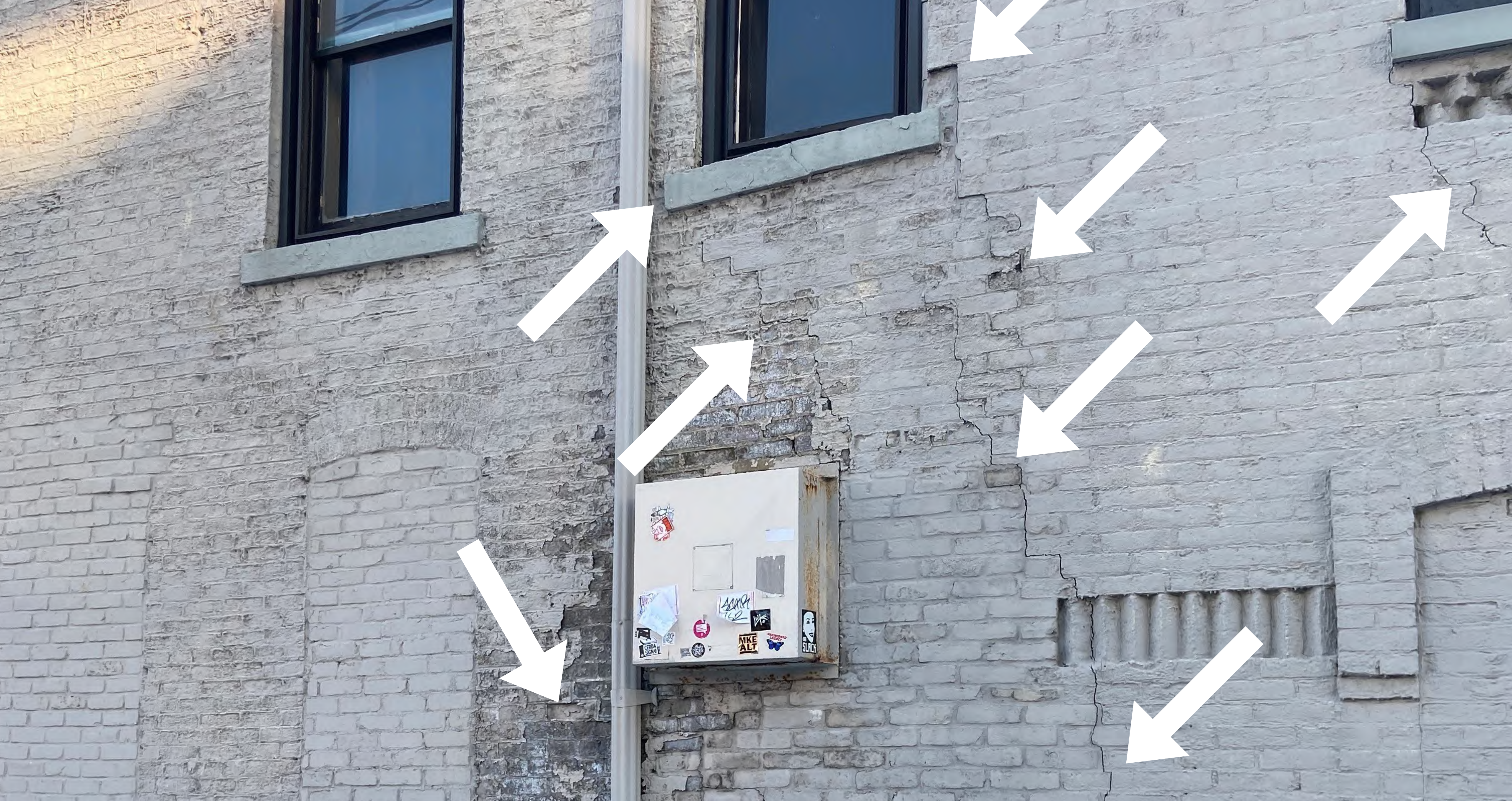
Brick Cracking and Deterioration
