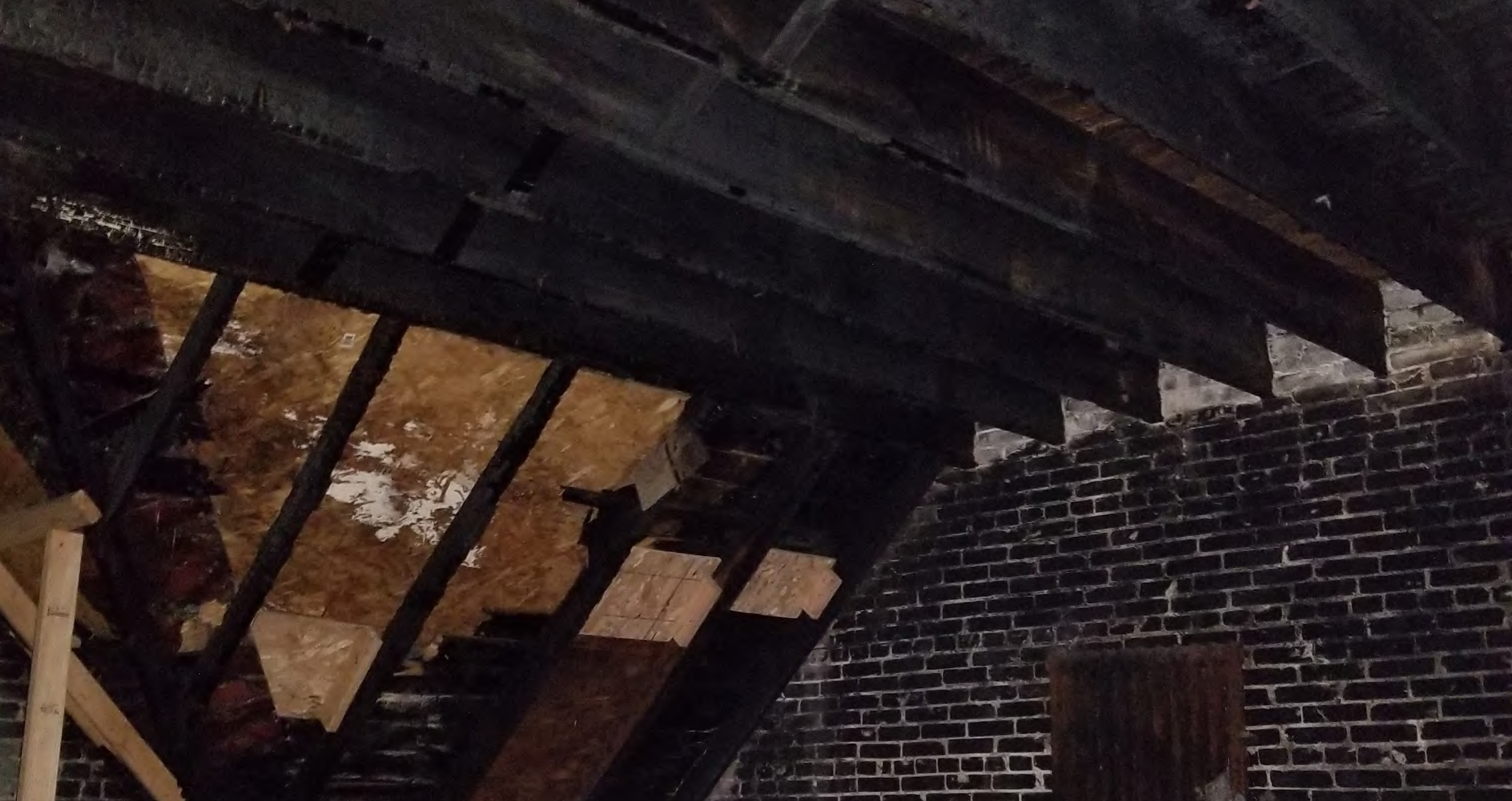
Roof - Structural Fire Damage
