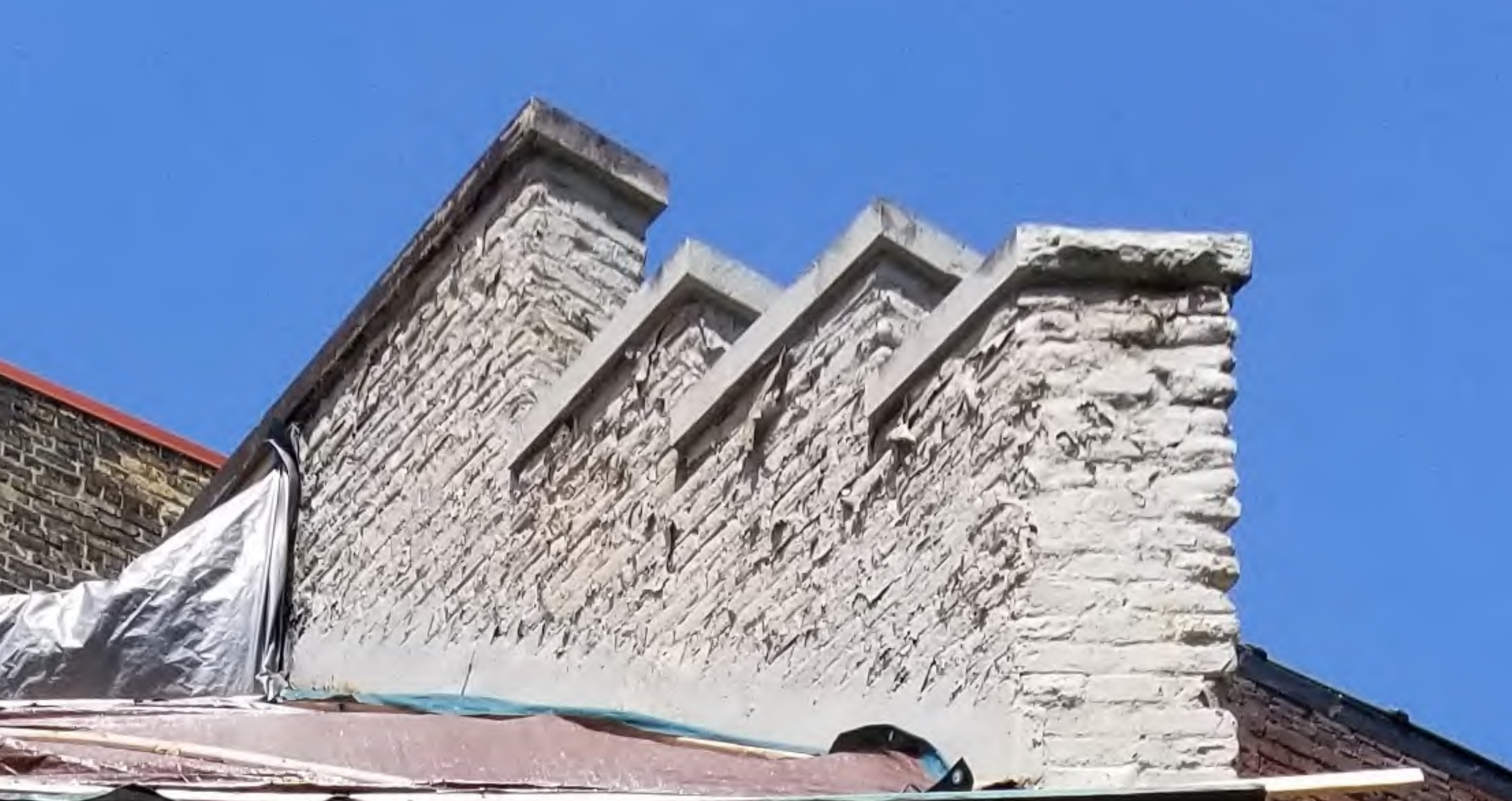
Structural Brick Deterioration
