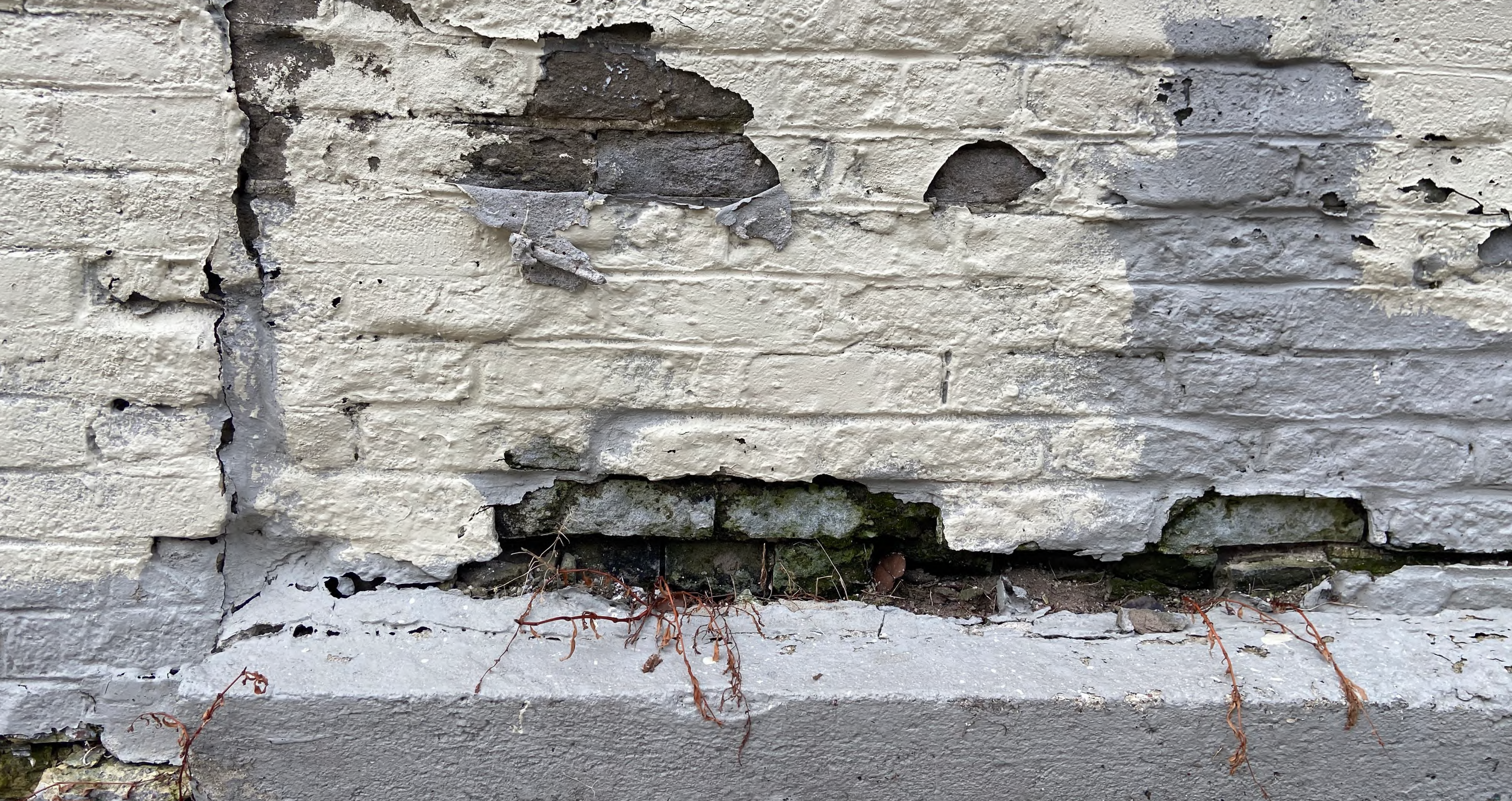
Structural Brick Deterioration
