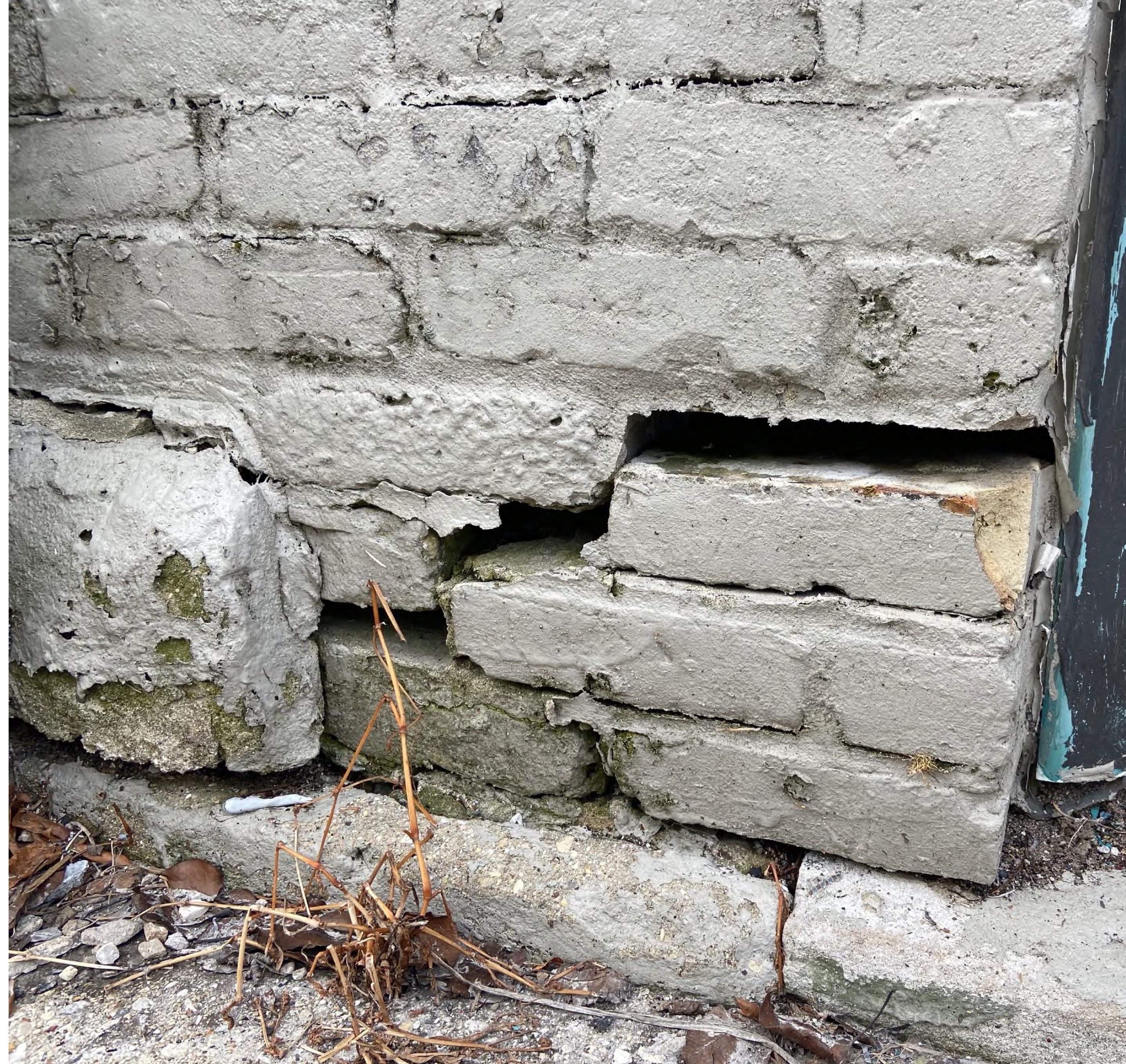
Structural Brick Deterioration
