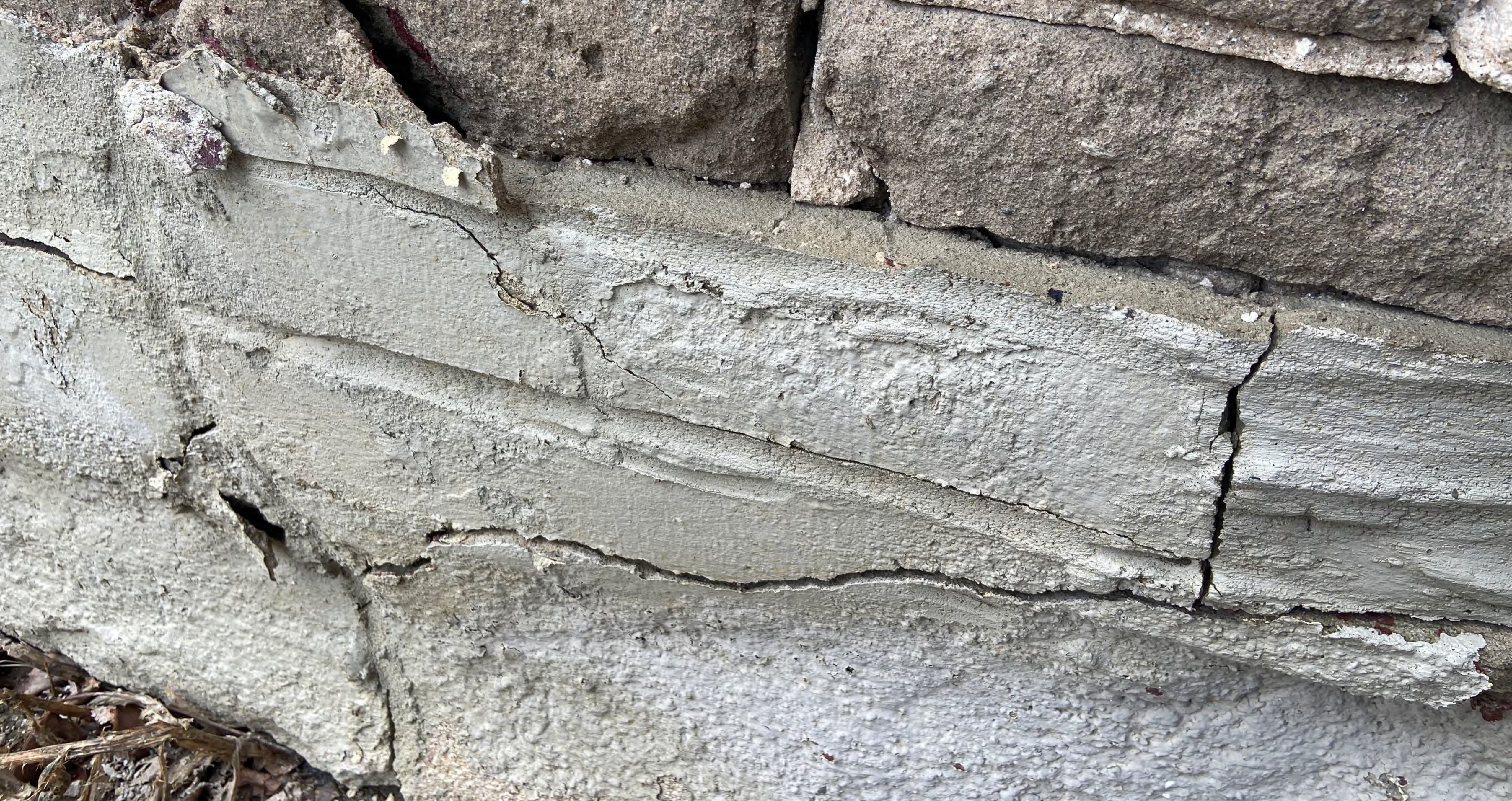
Structural Brick Deterioration
