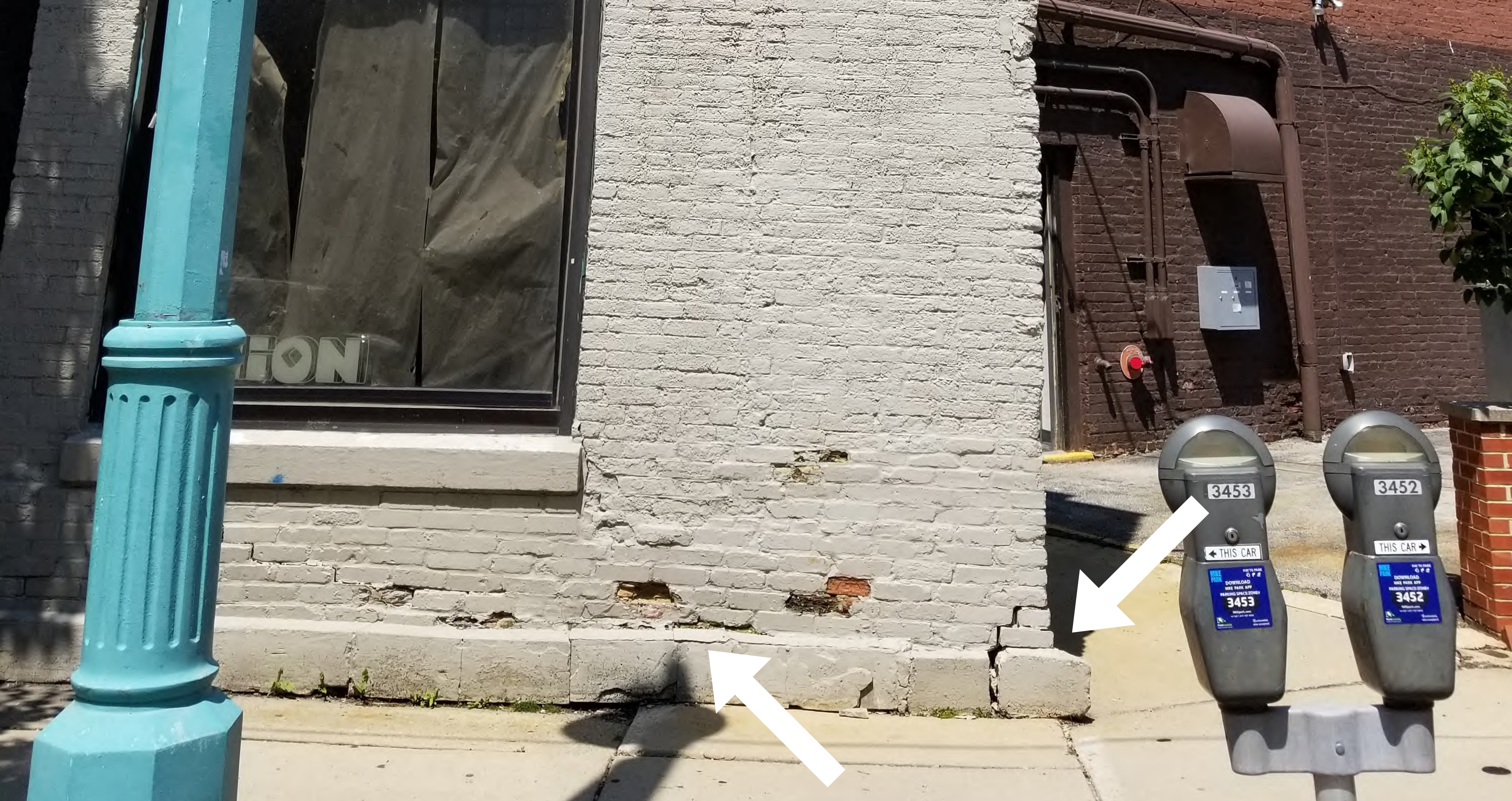
Structural Brick Deterioration
