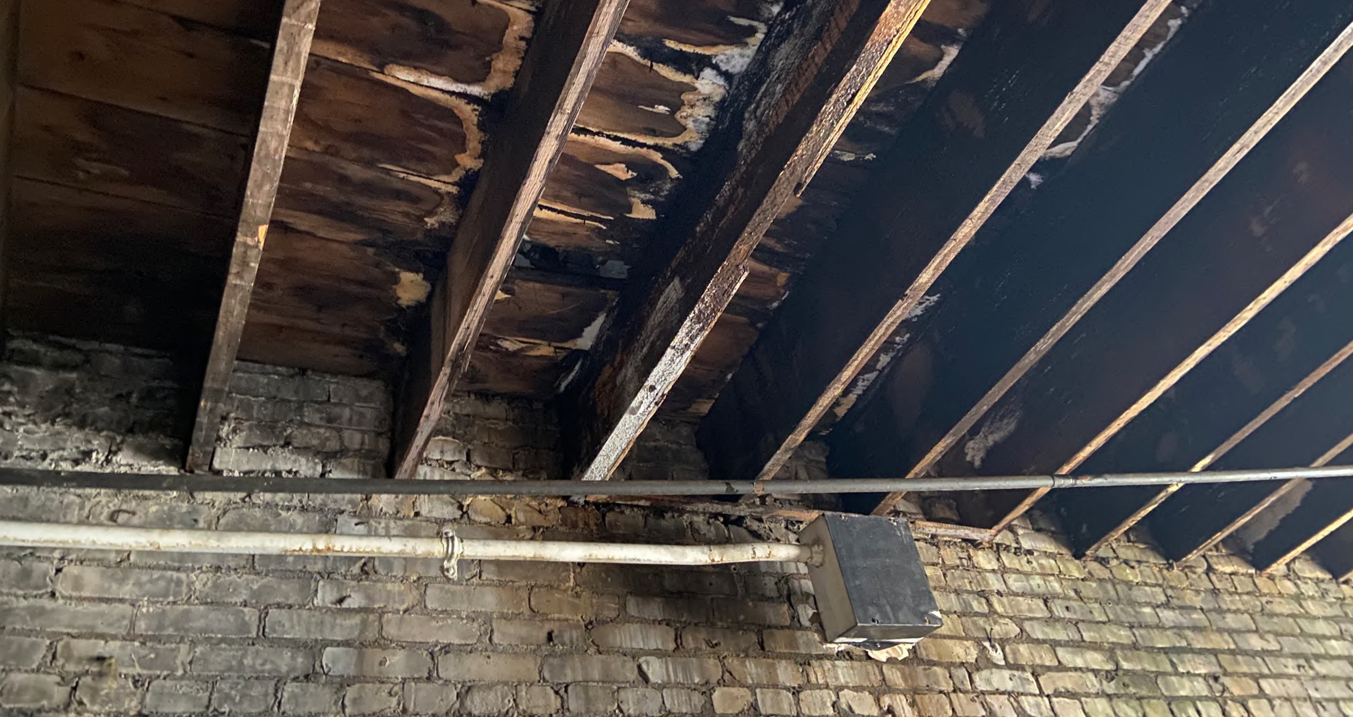
Floor - Structural Fire Damage
