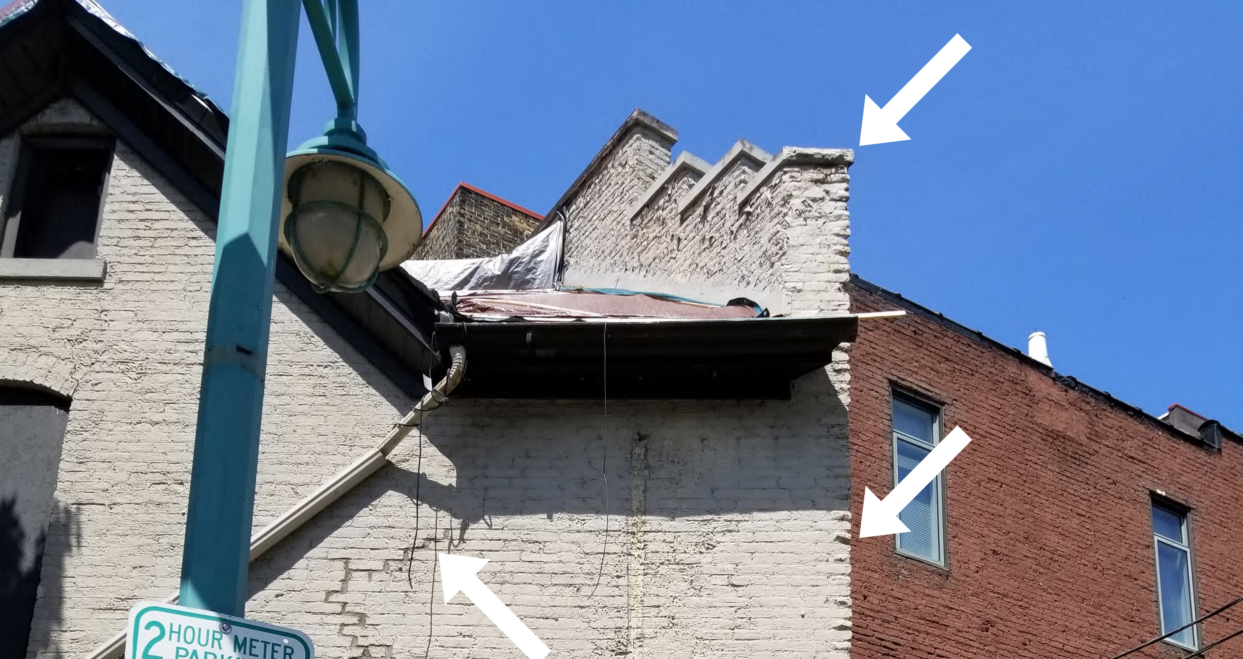
Structural Brick Deterioration
