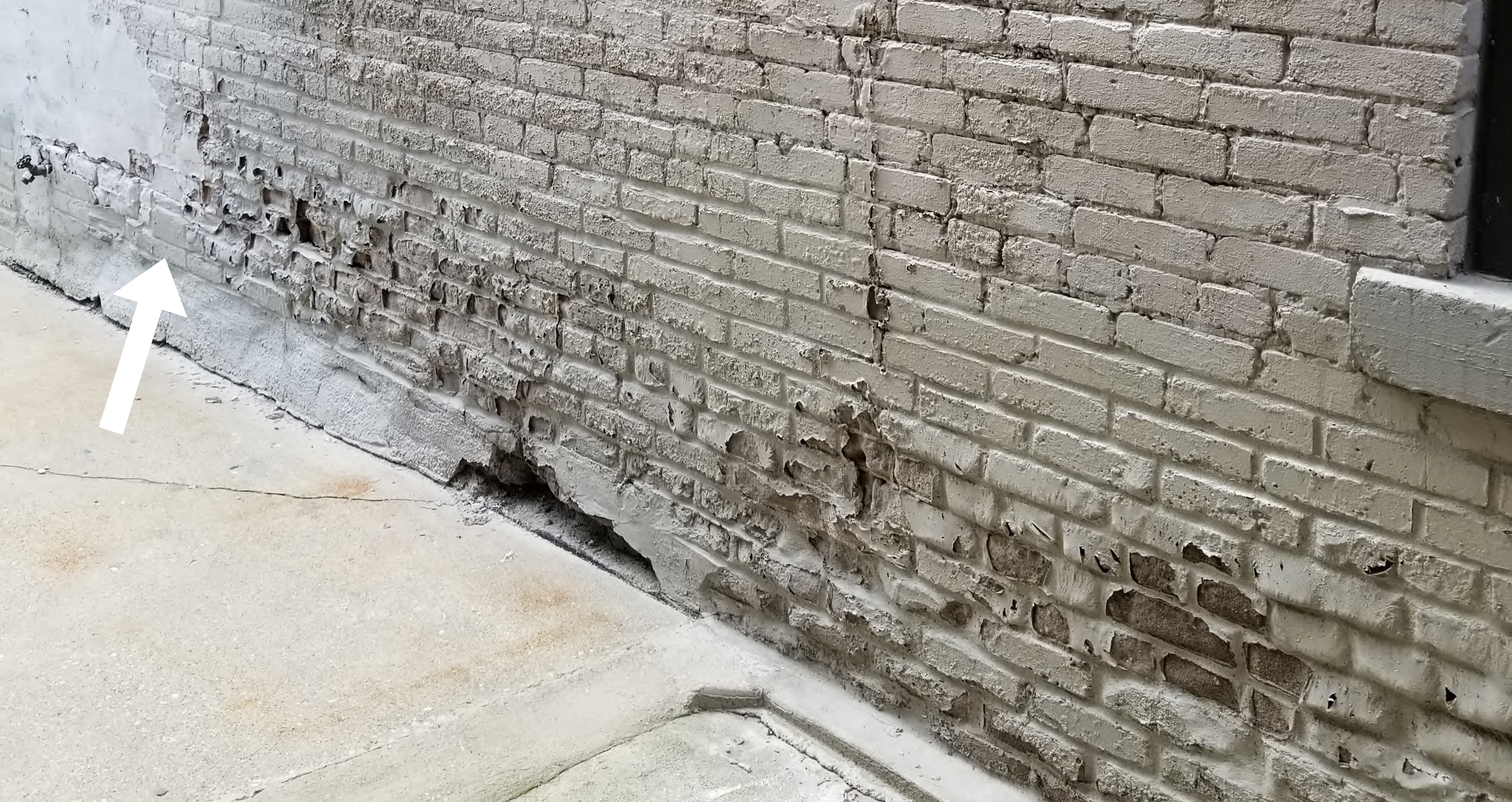
Structural Brick Deterioration
