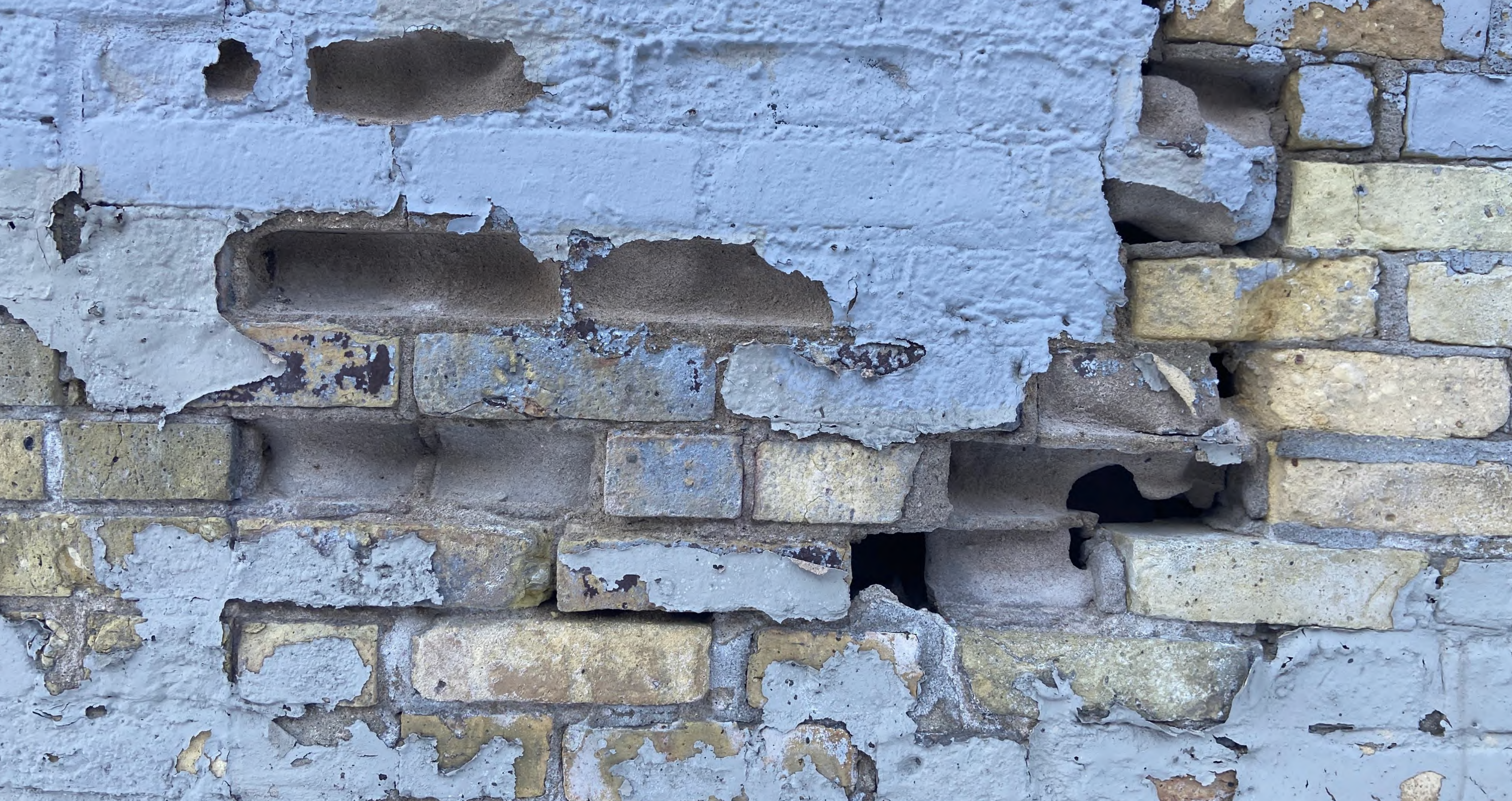
Structural Brick Deterioration
