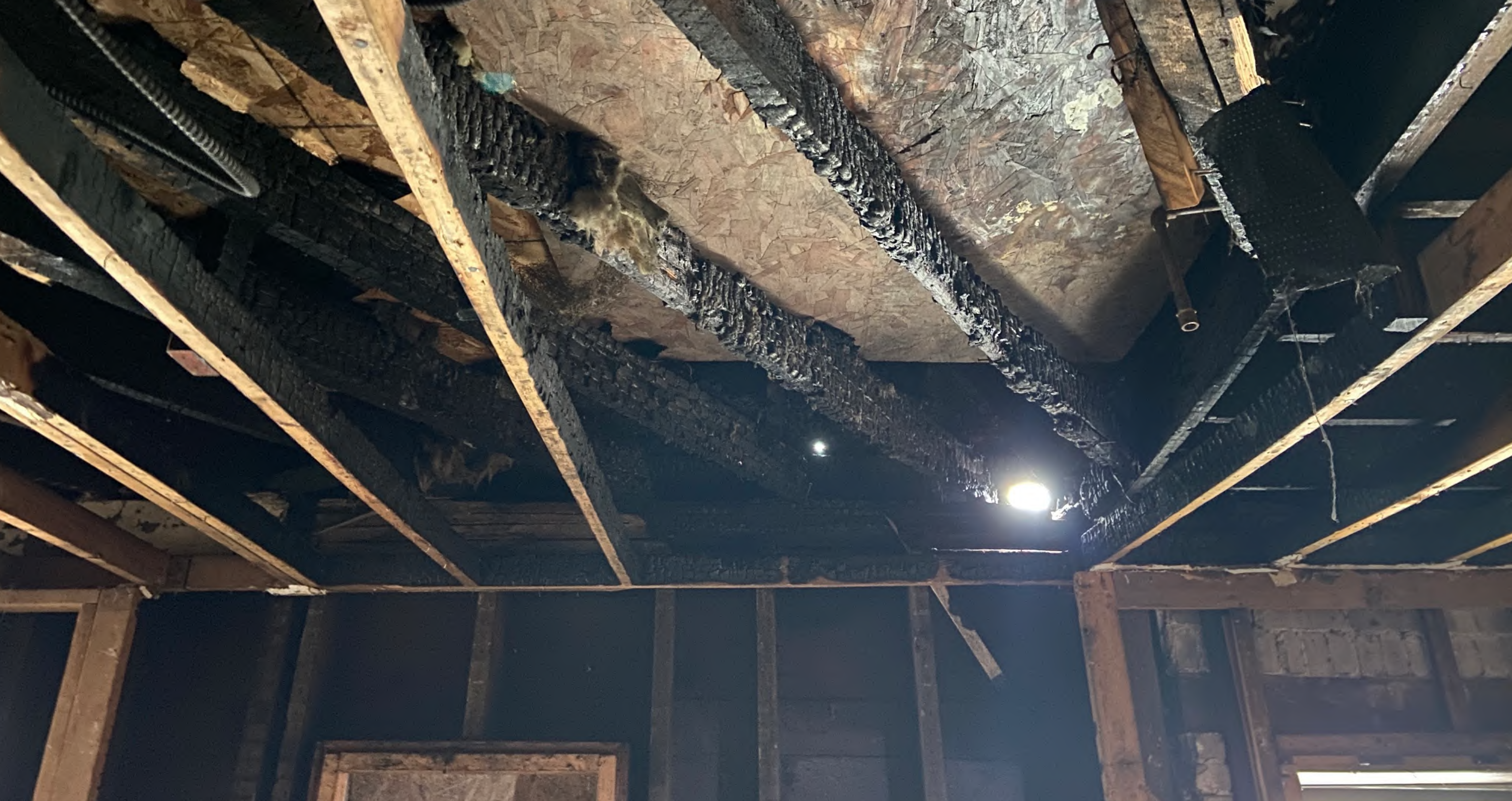
Roof - Structural Fire Damage
