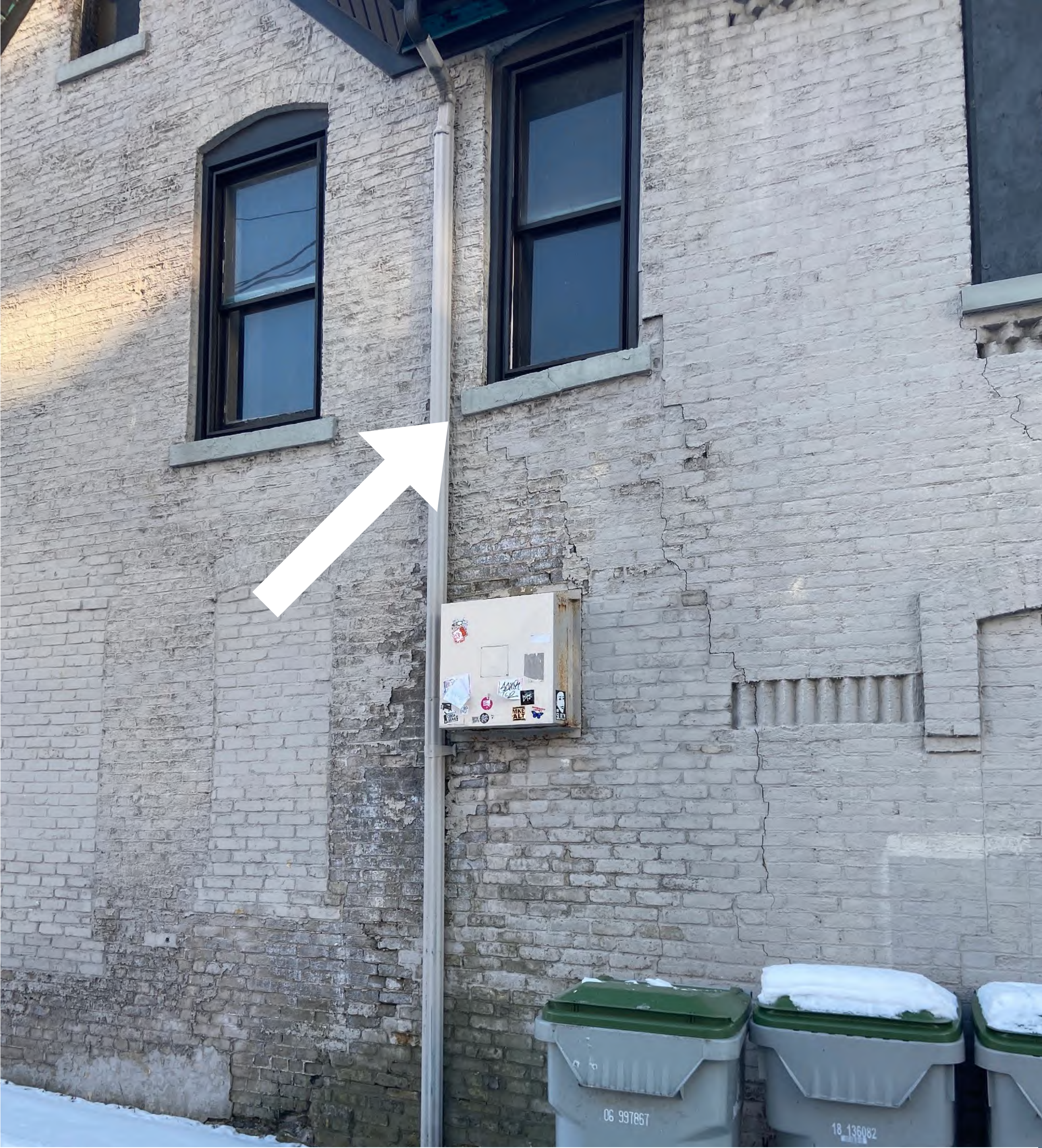
Brick Bowing and Settlement
