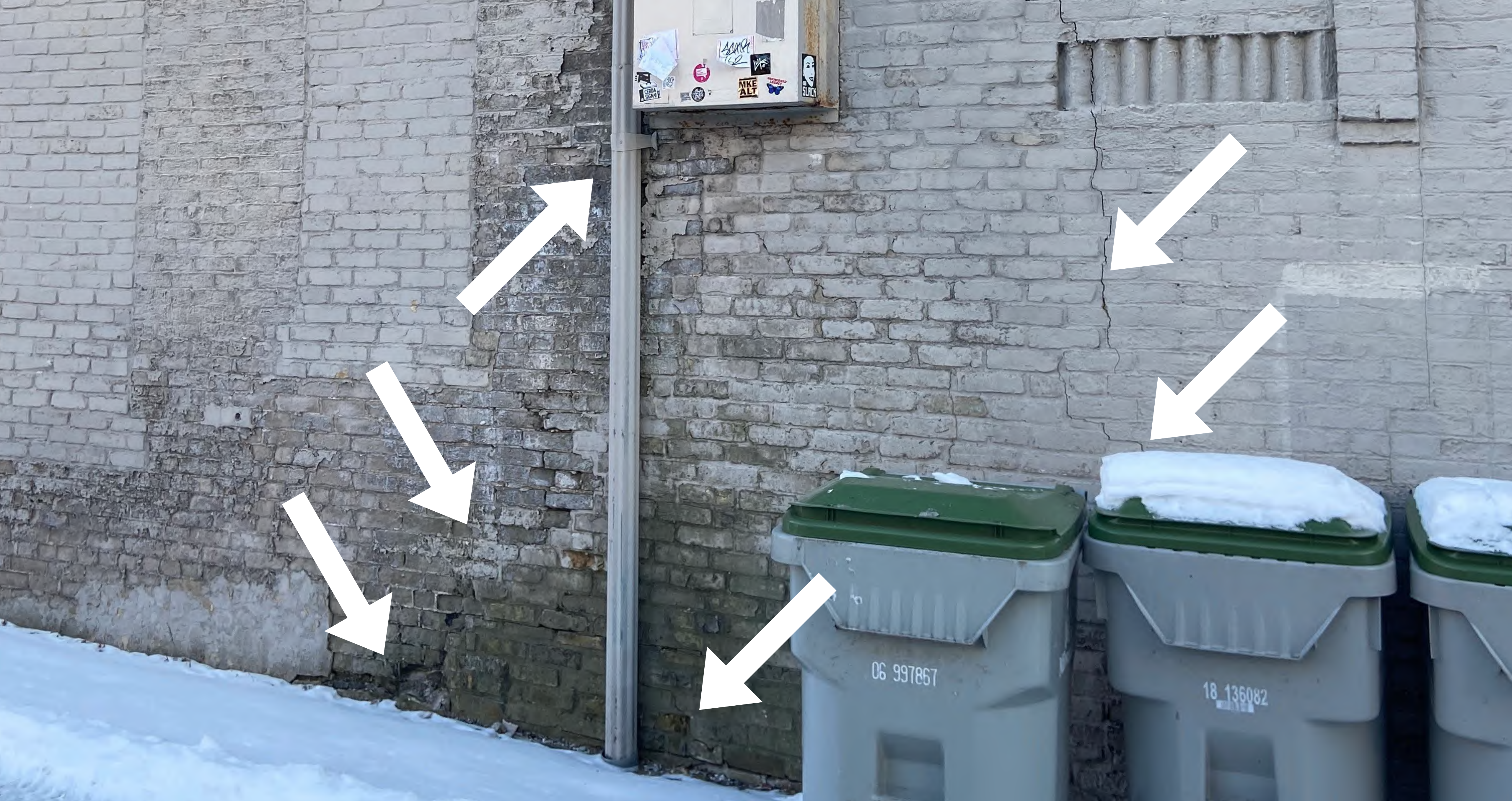
Brick Cracking and Deterioration
