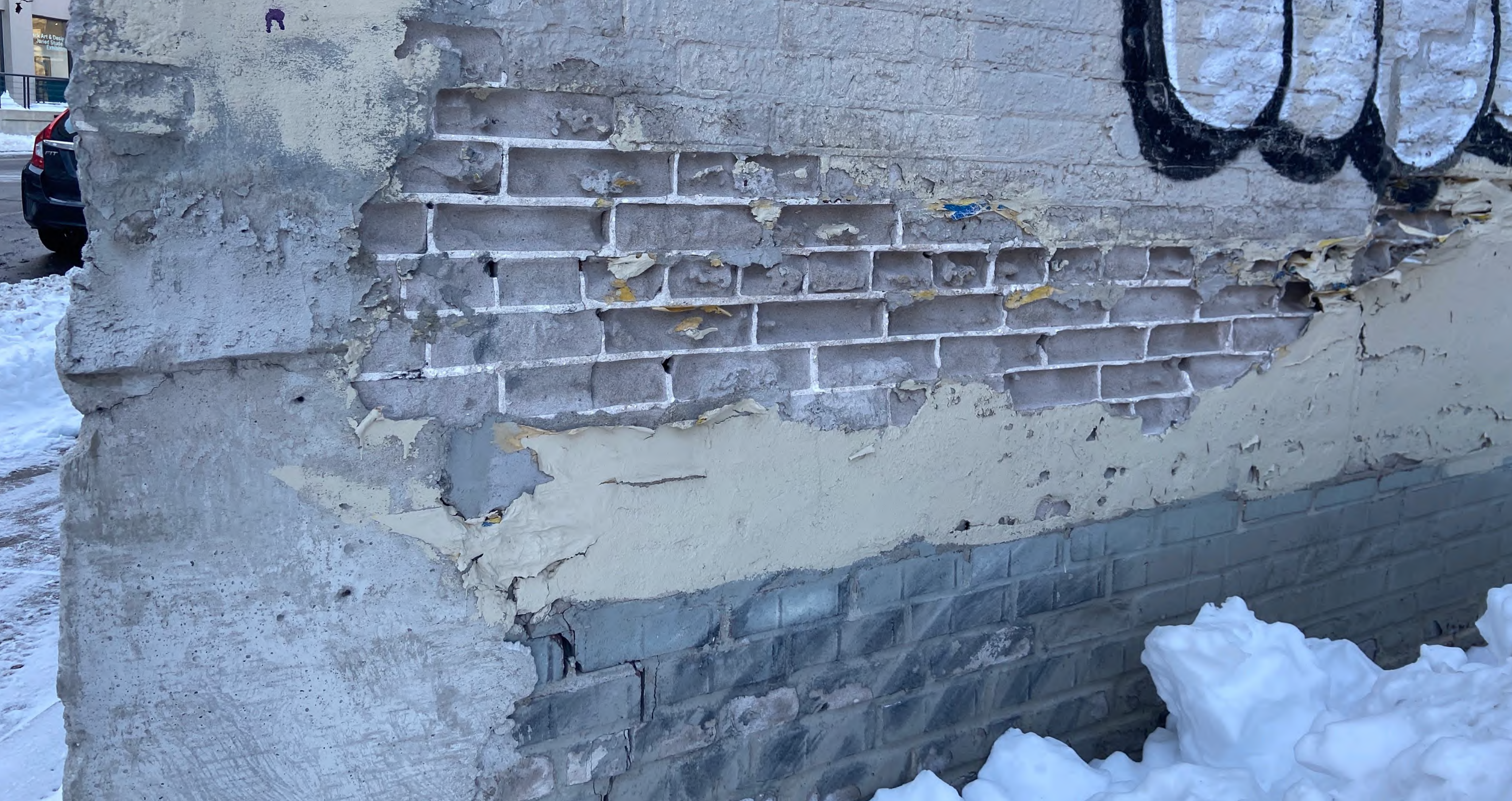
Structural Brick Deterioration
