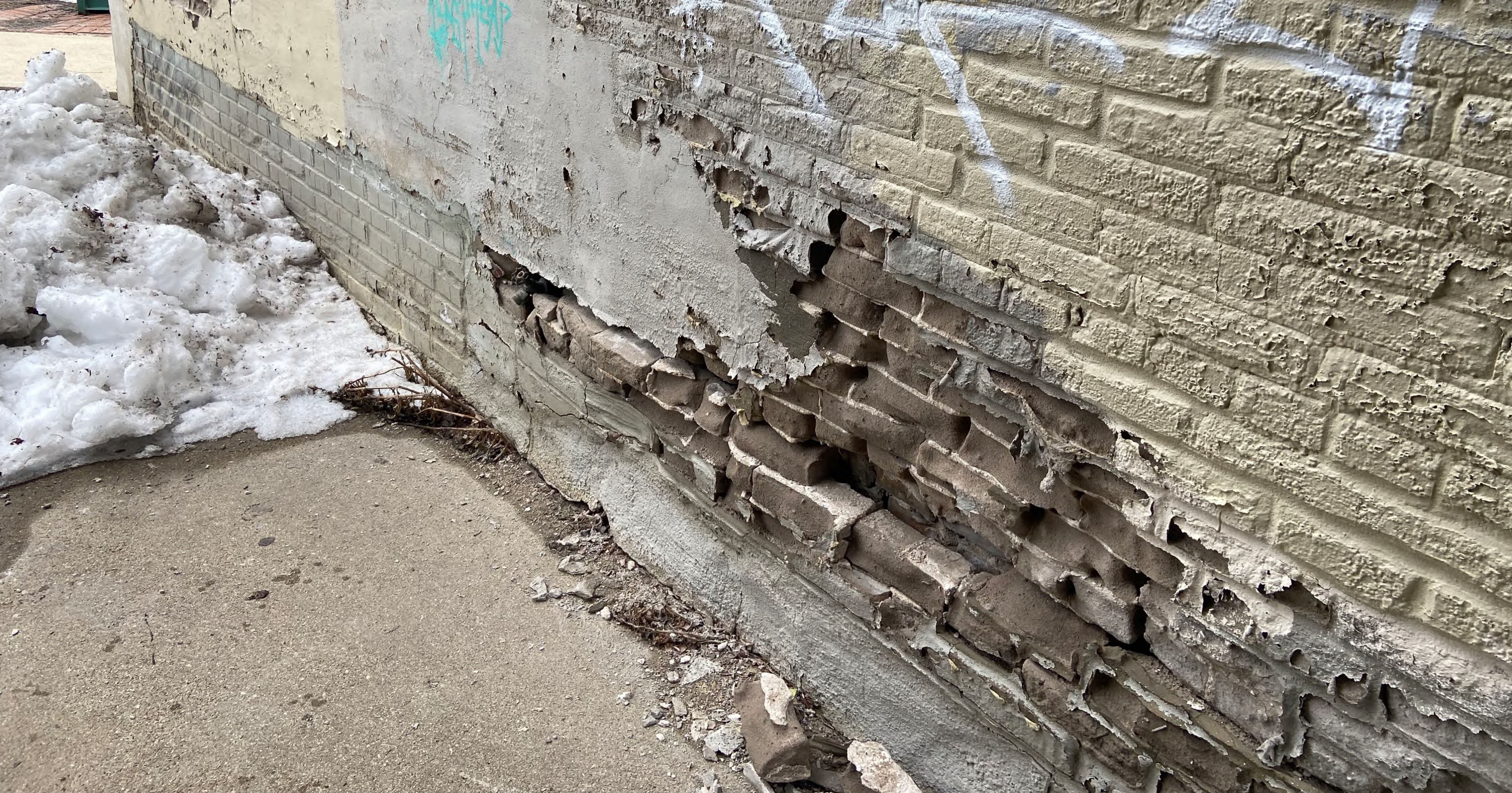
Structural Brick Deterioration
