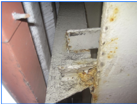
Paint finish with rust
