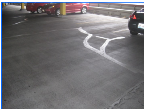
Membrane floor with prior repairs
