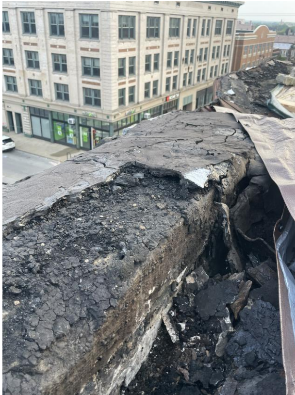
Typical location where new coping and flashing is required.
