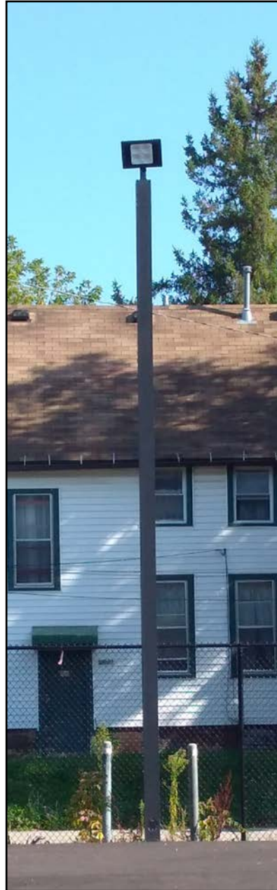
Parking lights: New north parking lot lighting installed at north perimeter adjacent to alley. Photo Taken: 08/30/17
