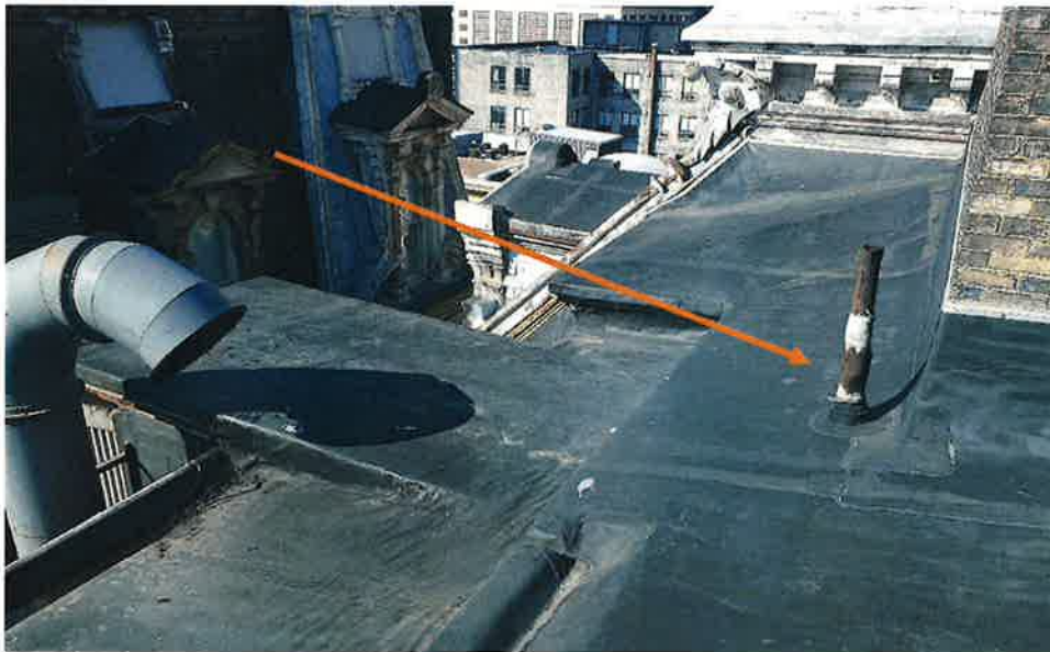
Figure 4: Penetrations will be reinforced in a 3-course method. Reference lines 11 and 17 in scope of work.
