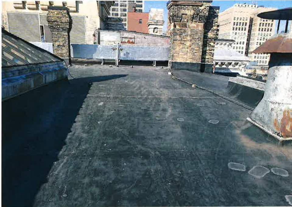
Figure 1: Field of roof will be cleaned, scrubbed with detergent, and pressure washed. Reference line 3 in the scope of work.
