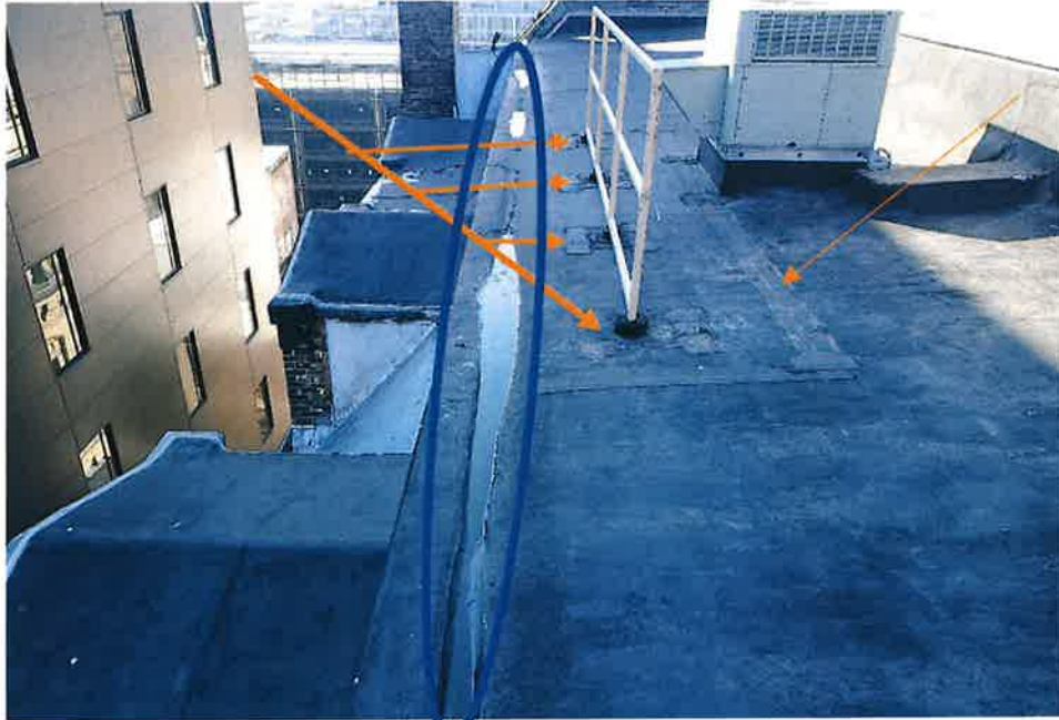
Figure 5: Seams and base of railing will be reinforced. Reference lines 11 and 17 in scope of work.
