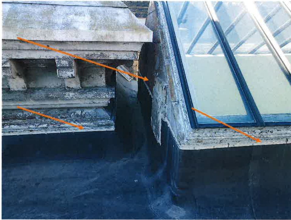
Figure 3: Term-bar will be reinforced with trowel grade and then top coated. Silicone will run about two inches above termination bar. Reference lines 11, 12, and 18 in scope of work.
