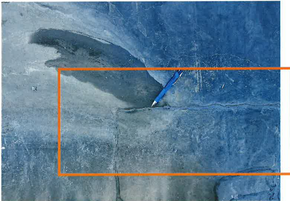
Figure 2: All seams will be treated in a 3 or 4-course fashion. 4-course example Trowel Grade, Fleece, Trowel Grade, topcoat. Reference line 10 in the scope of work.
