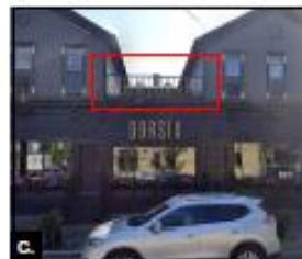
New Decorative Wood Railings: Wood railings, posts, rails, balusters, railing caps and finishes to match existing wood railing located above Dorcia sign on the North face of the building.
