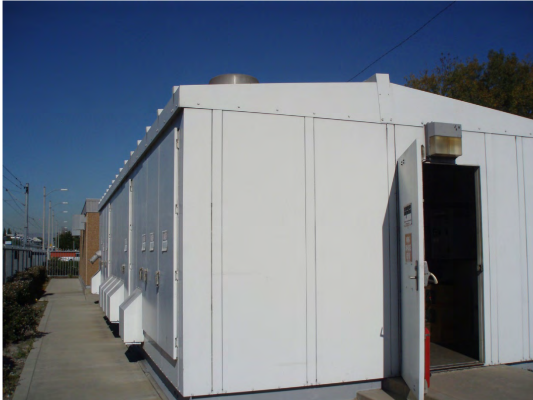
Figure 43: Example Photo of a Power Substation
