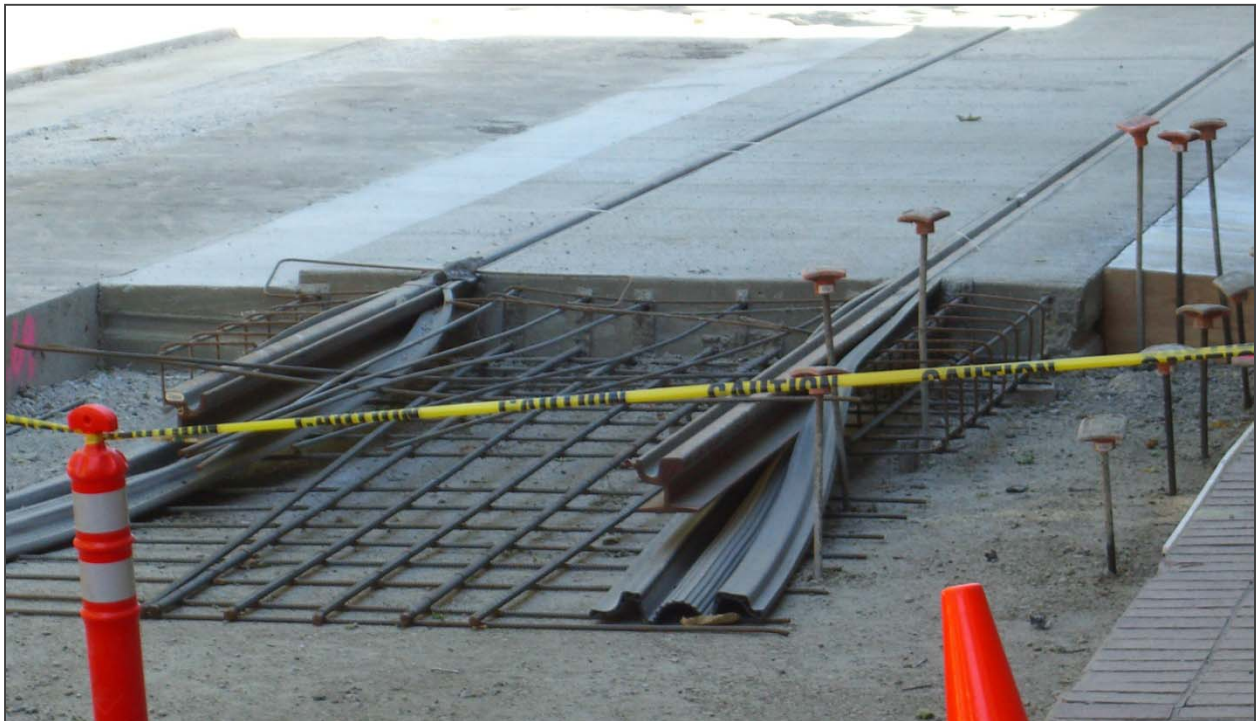
This is an example of a streetcar track being constructed in Portland, Oregon that shows how the rubber boot is wrapped around the rail to reduce noise, vibration and stray current. Image: City of Milwaukee.
