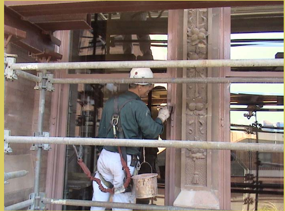
Painting the exterior of the window frame after the glass has been replaced on the 3 rd floor.
