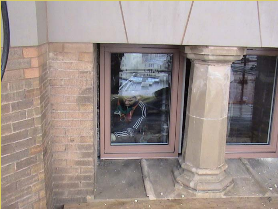
Installation of insulated windows on the 9 th floor of the south tower.
